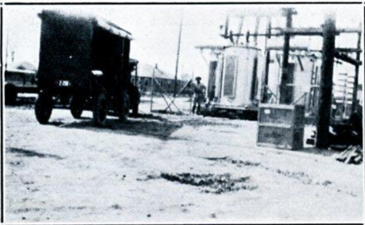
Oil filter trailer hooked up to transformer.
