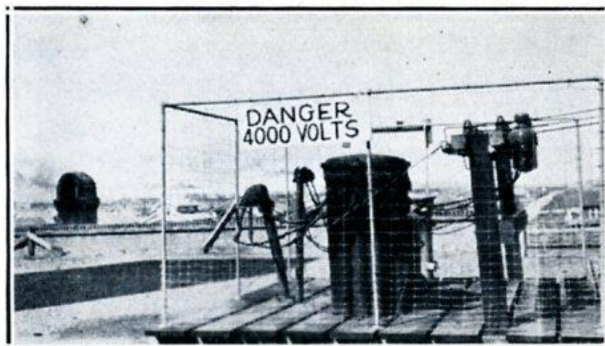
Reworked transformer bank at Franklin School, Port Arthur. This is a fine bit of work by Sub-Foreman Adams and his line crew.
