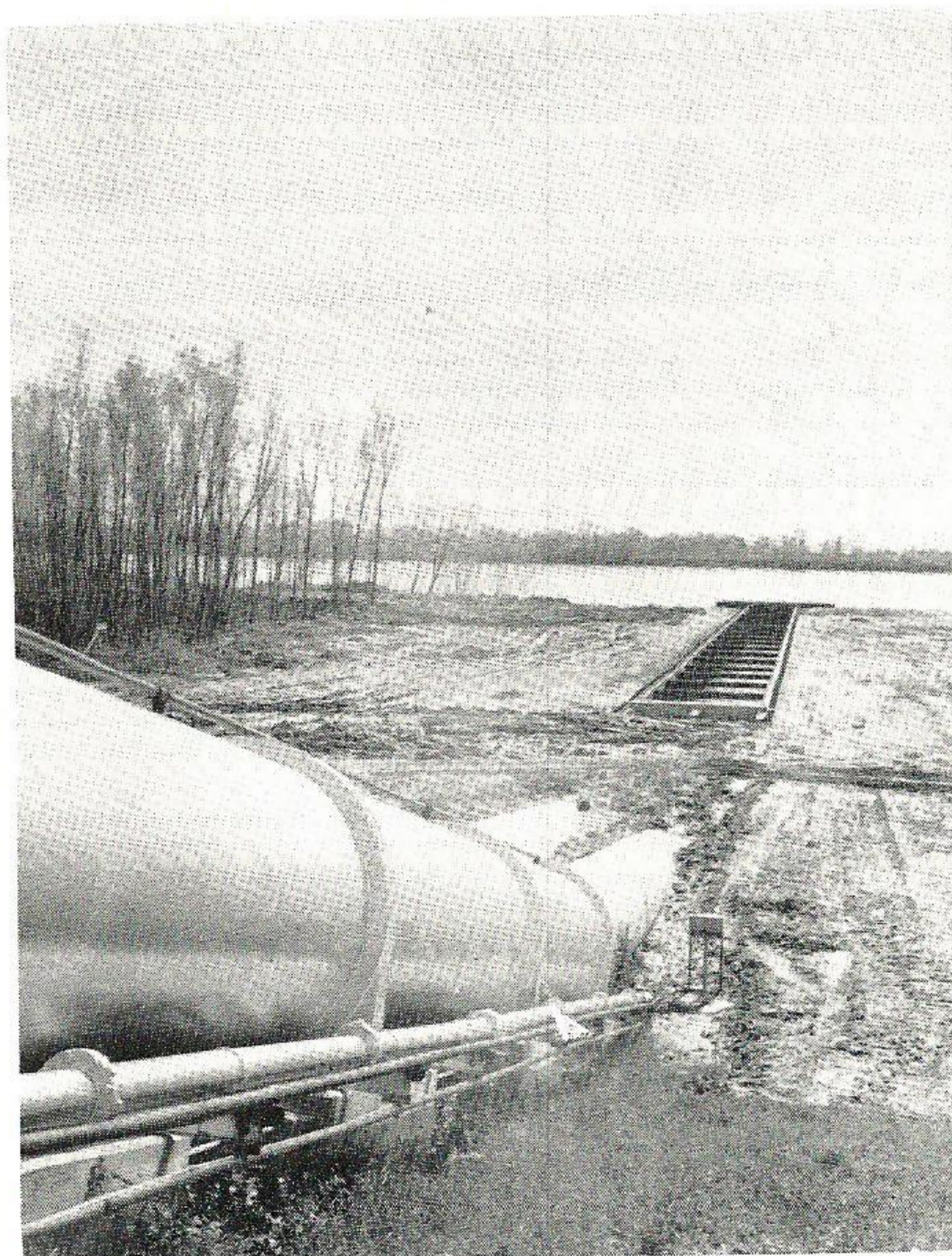
Huge water pipes run over the levee into the Mississippi River, to carry cooling circulating water to and from the boilers.
