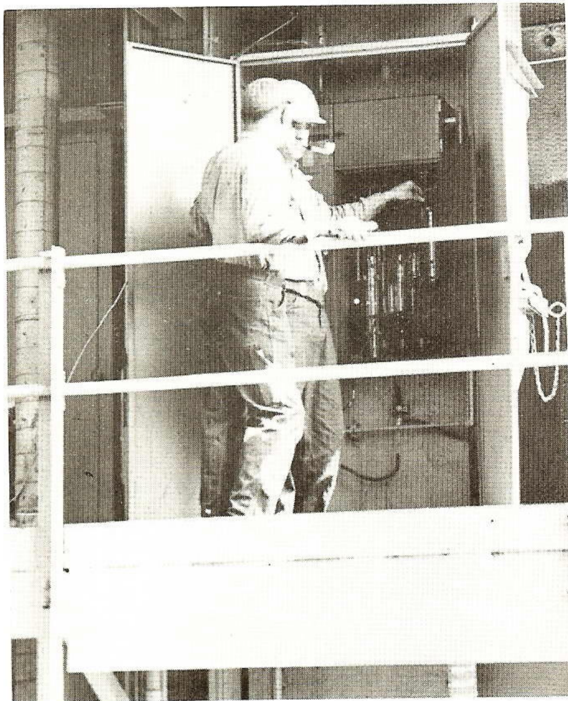
CONSULTATION. Wayne talks to George Naquin, first class repairman, as he is checking an O 2 Analyzer, which analyzes the amount of oxygen in the gas in the furnace. This tells the fireman how much excess air is in the boilers.
