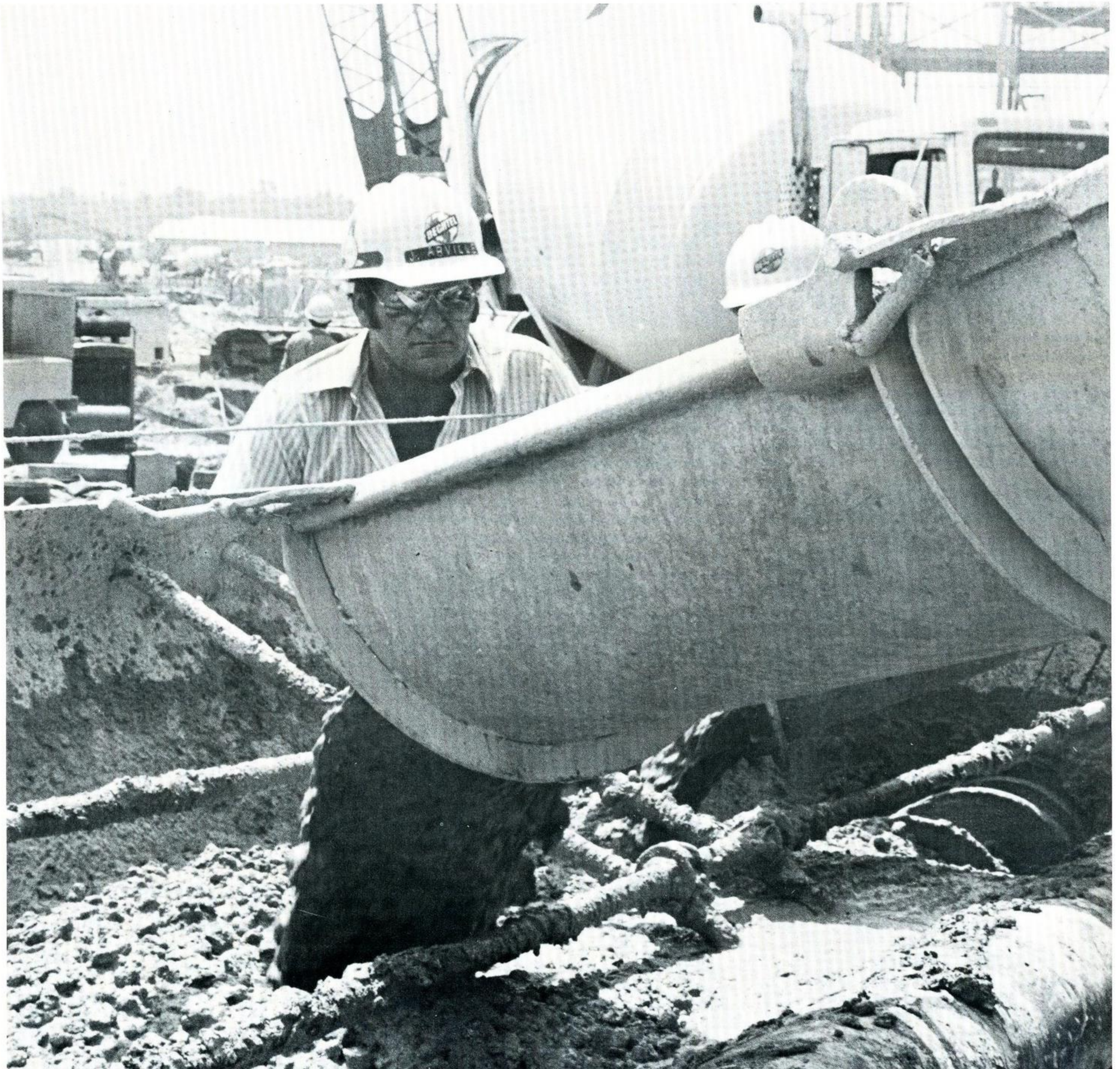
About 3300 yards of concrete were required to create the eight-foot thick foundation for the massive Nelson 6 stack.
