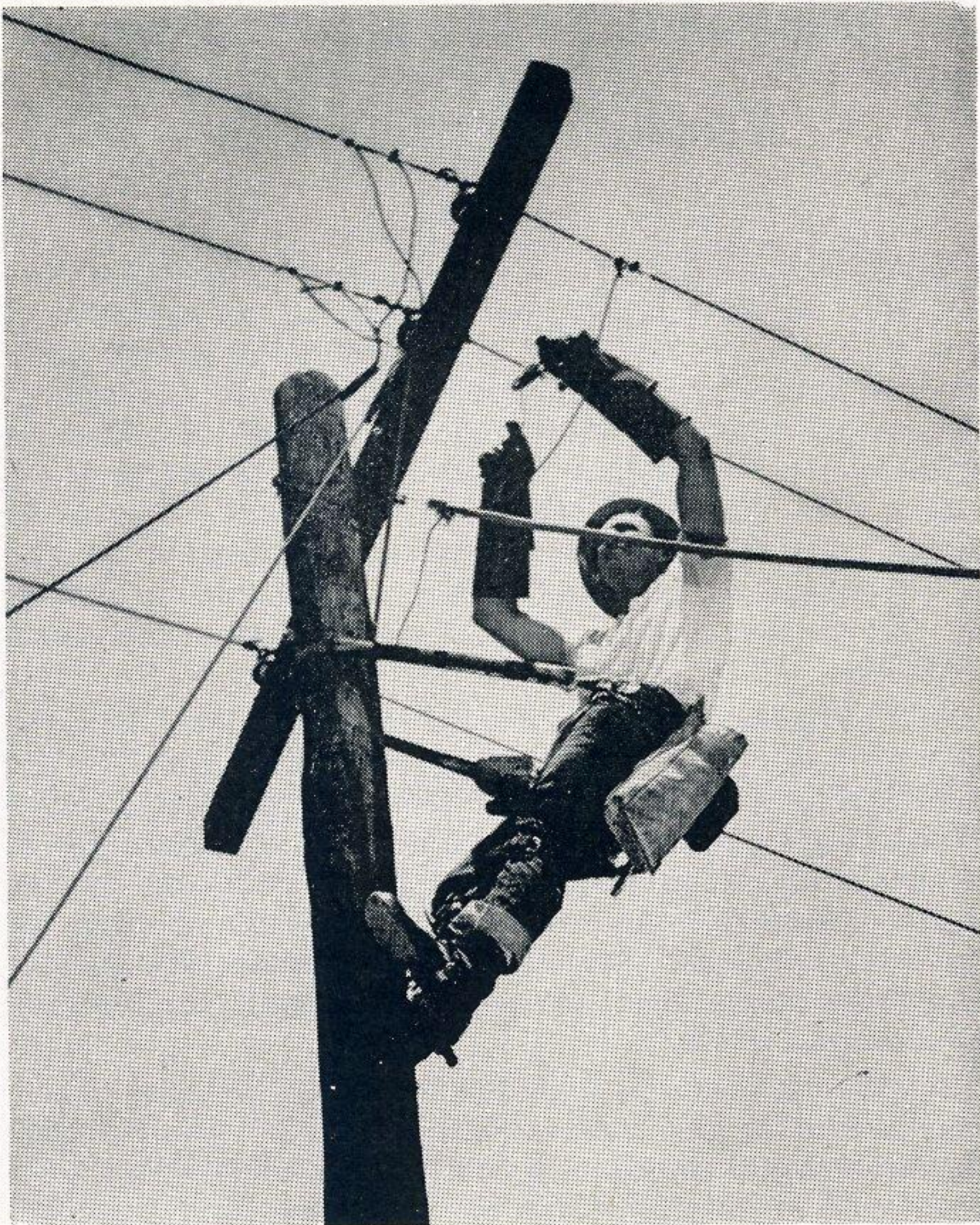
Beaumont lineman Lanclos "cuts out" a burning home.
