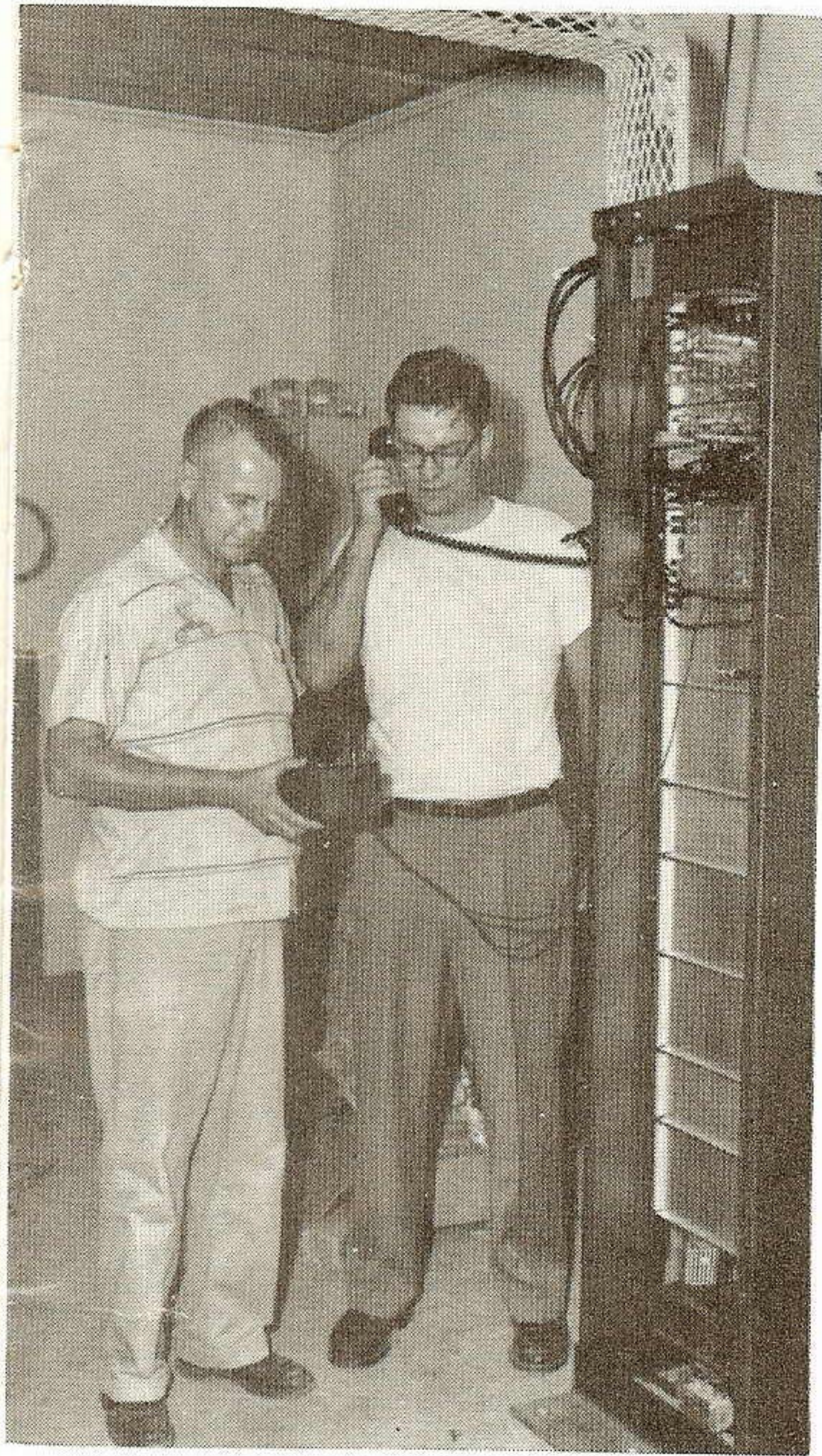
William Tucker, Baton Rouge Relay Department, and William Hack, Beaumont Relay Department, test the microwave transmitting and receiving equipment at Amelia Bulk.
