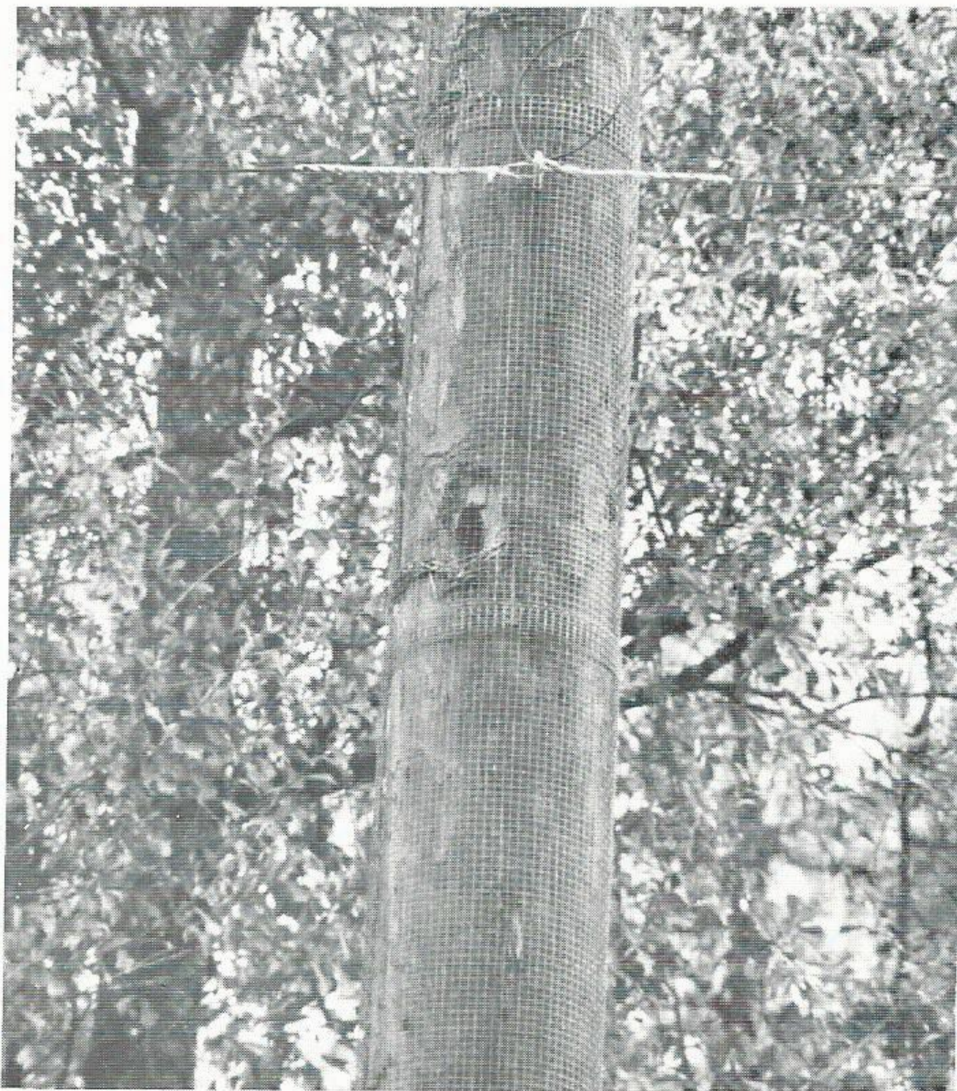
Wire mesh is being used to protect the poles and this seems to be the most effective preventive measure to date.
