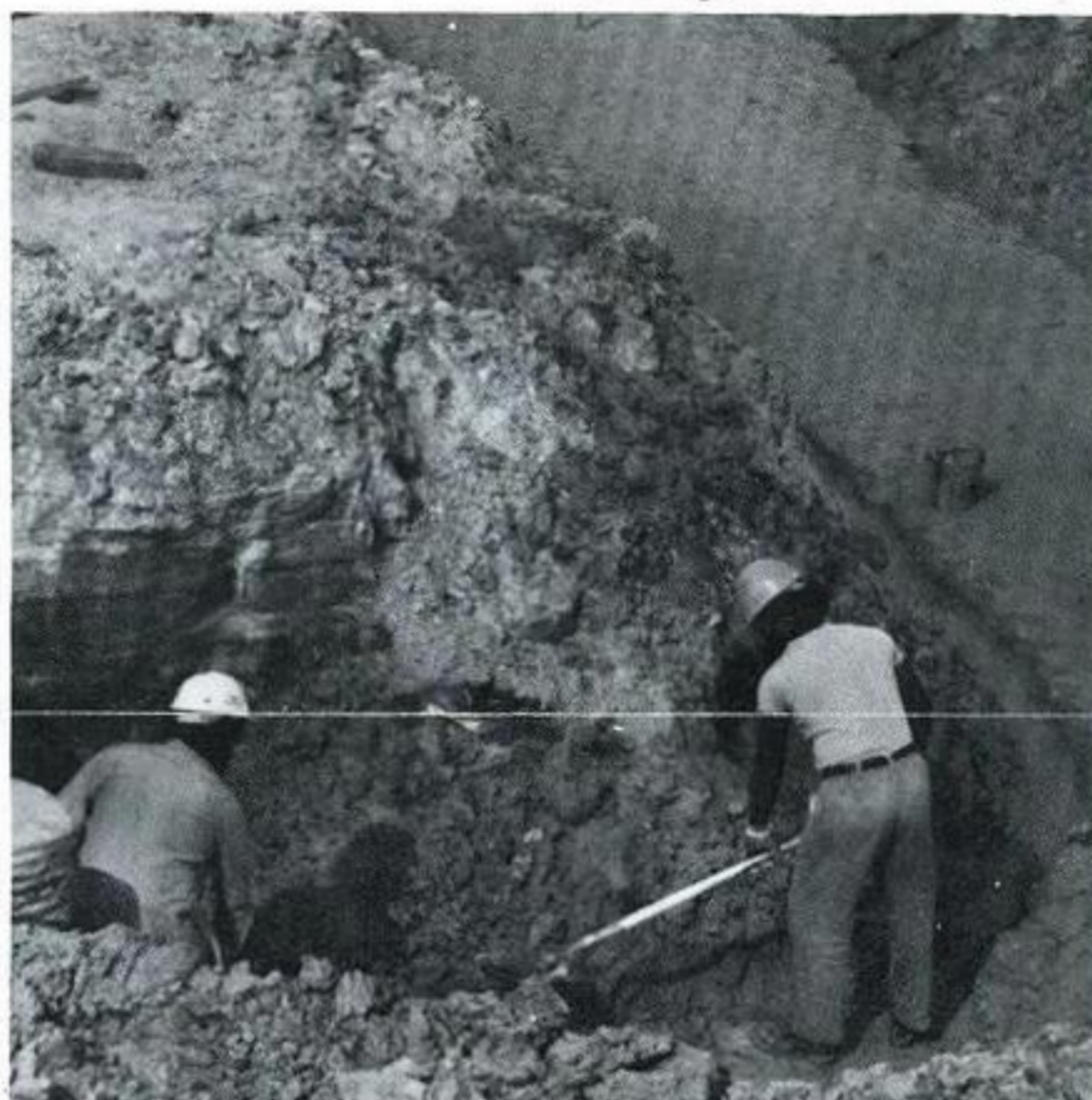
One of the bright spots for GSU during 1978 was the start of construction on Nelson #6, the company's first coal-fired unit. The men above are shown working on the excavation and placement of the sand bedding for the unit's 78-foot circulating water line.
