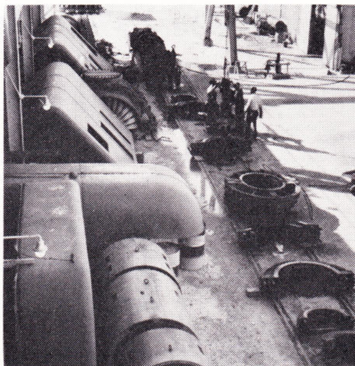
Looking down at some of the parts of the turbo-generator, an idea of the tedious work involved in dismantling this giant can be visualized. Larger parts at left are the turbine housing.
