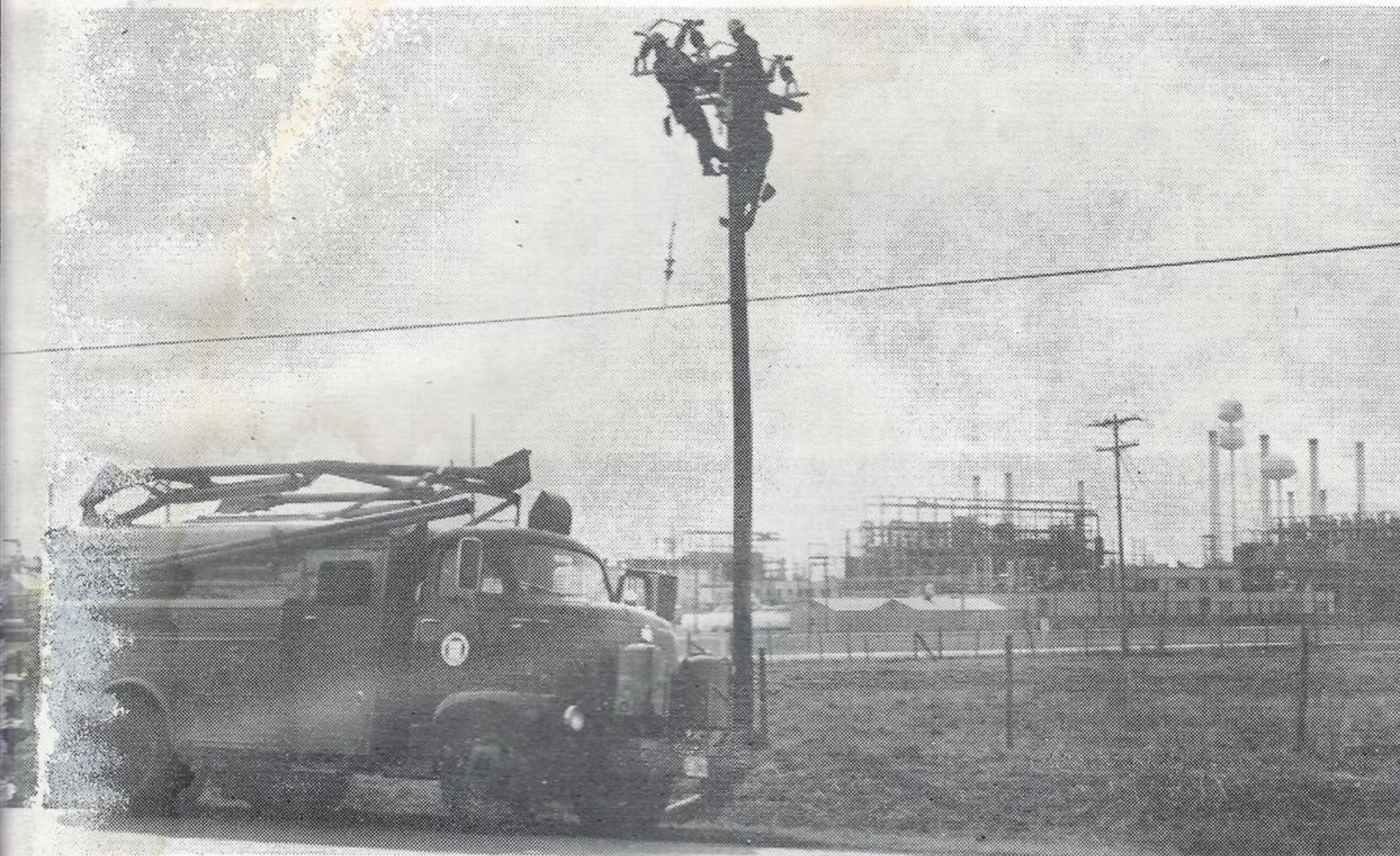
Lineman and linework are important to our Company's expansion program. These Gulf Staters are underbuilding a fourth feeder line near Chemical Row, Orange. Completion of the line will assure a more dependable supply of electricity for those vital petro-chemical companies.
