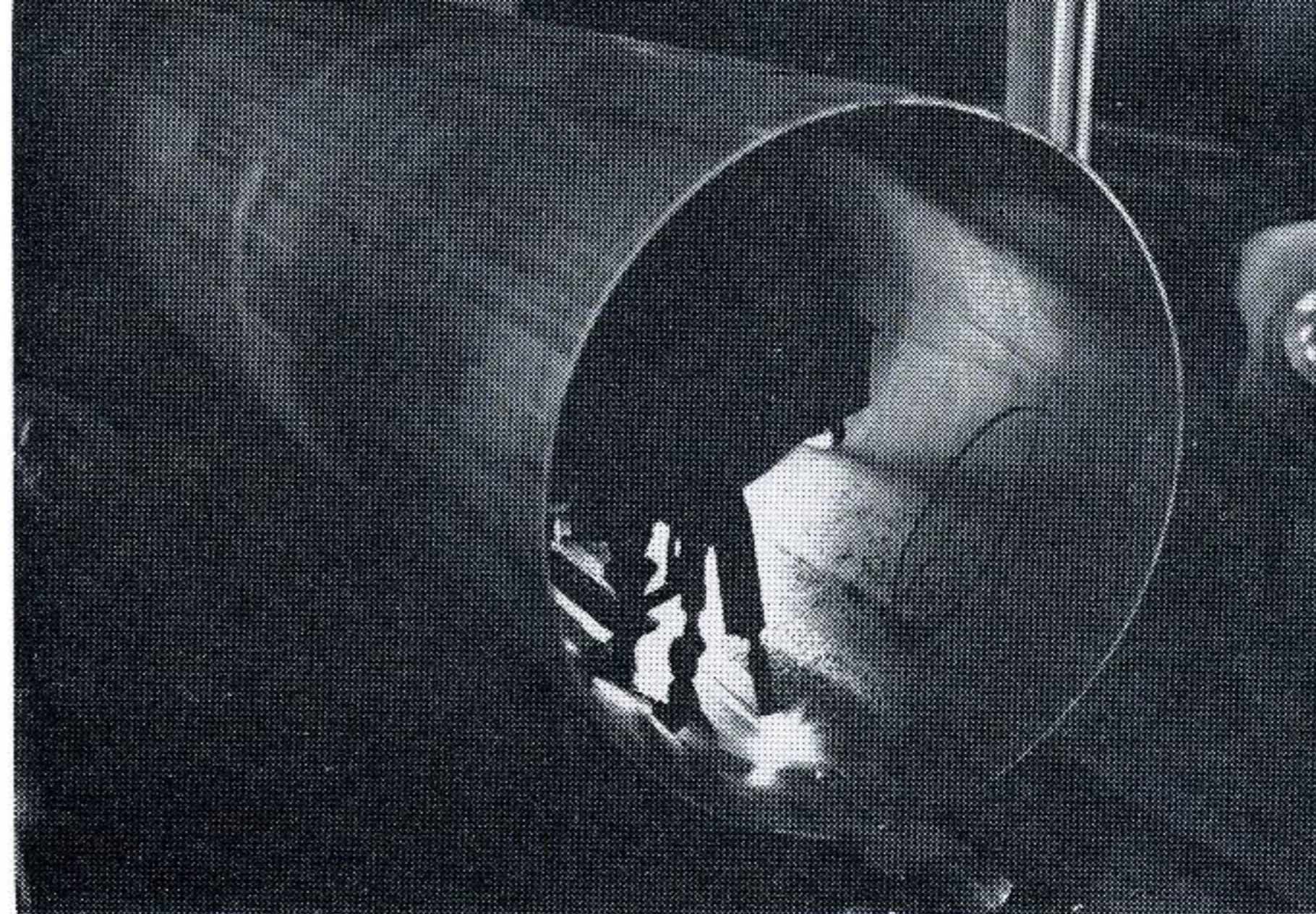
Welding pipe in this Orange plant is done using service furnished by our Company
