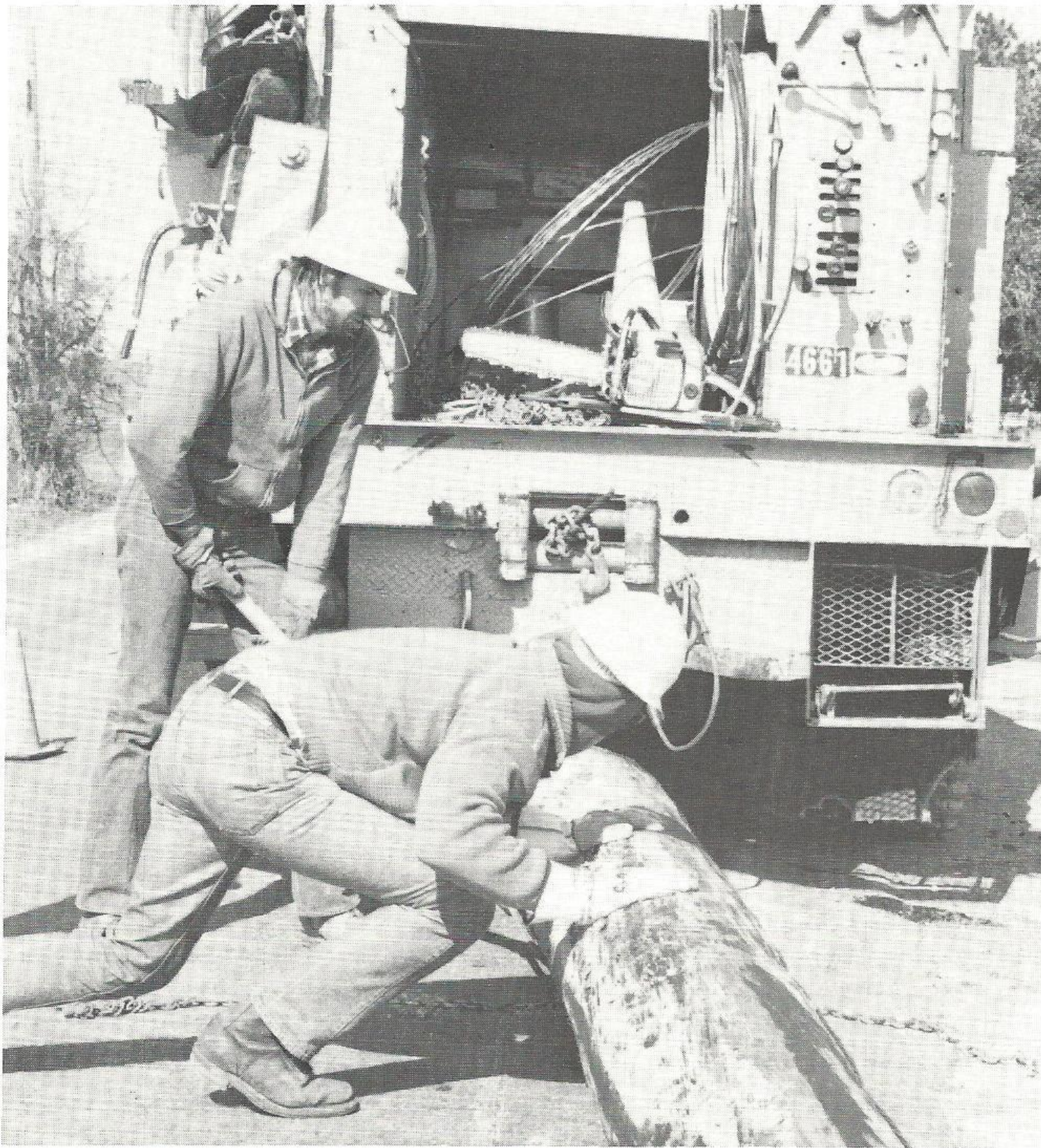
Dennis Delk (background), apprentice, and Albert Clay, lineman-2nd class, roll a utility pole into position for raising.
