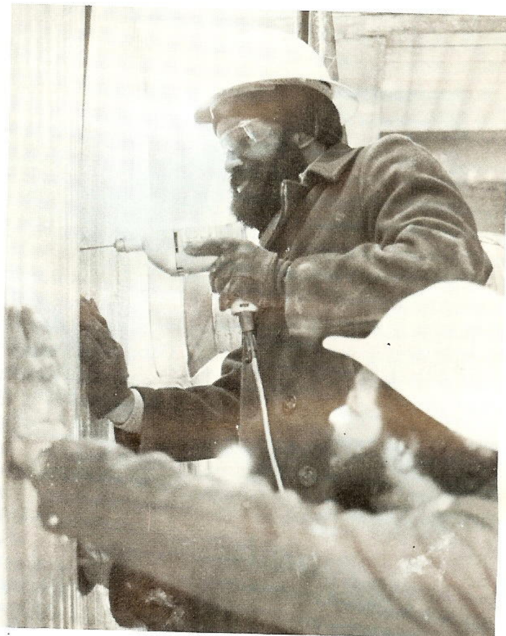
Earnest Rucker (standing), repairman-1st class, and Horace Braziel, equipment operator, install a shield to protect the plant from December's bitter winter winds.
