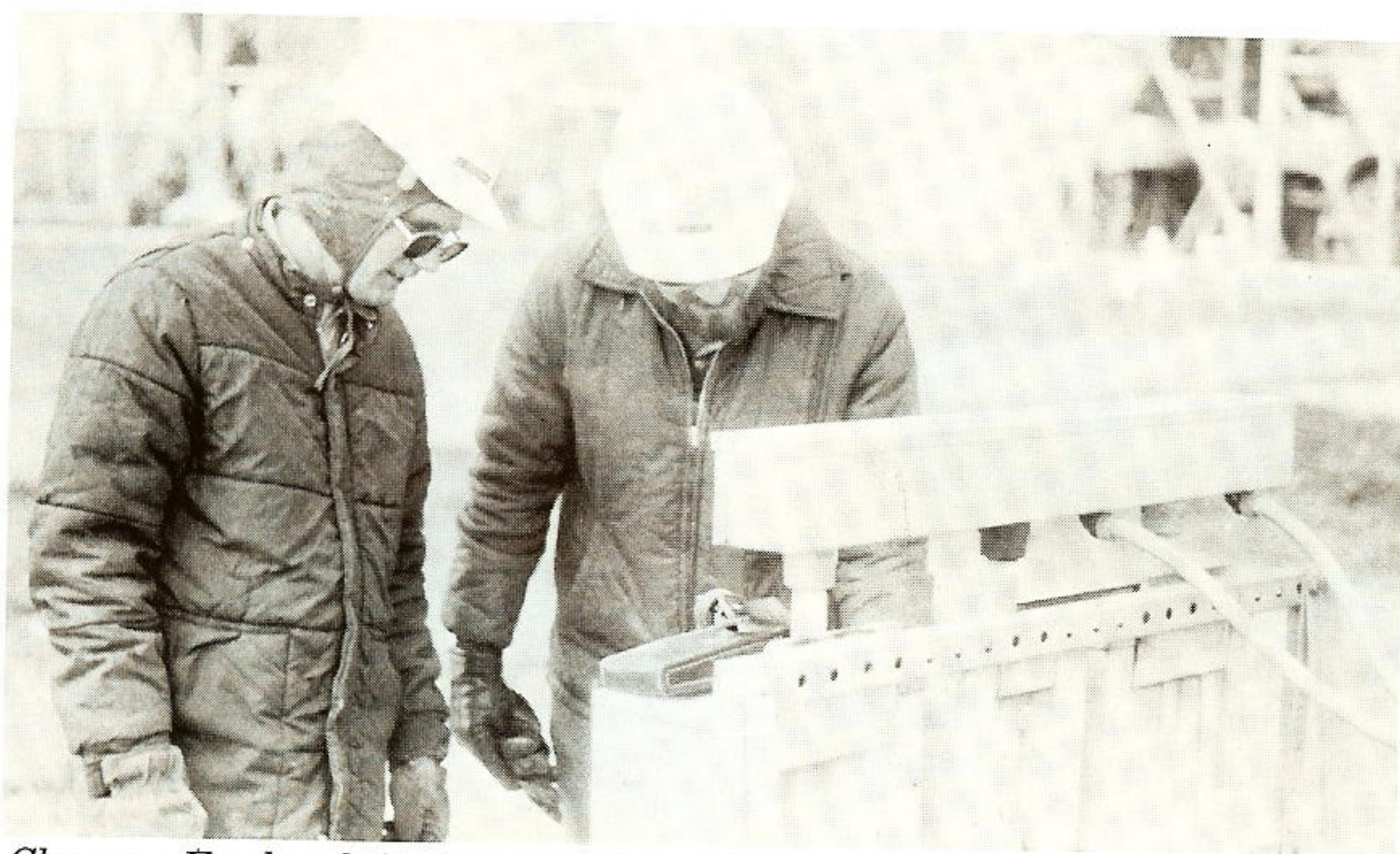
Clarence Fowler (left), test technician-1st class, and Cliff Jones, master electrician, repair a breaker shorted out by ants.
