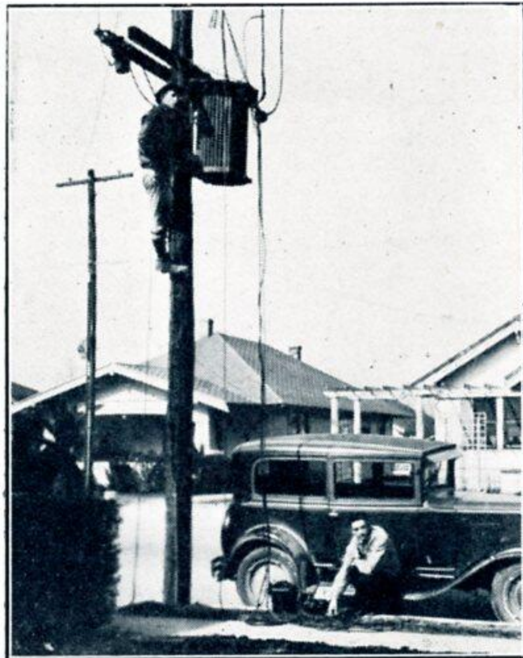
G. B. Oglesbee, lineman and R. O. Hopkins, distribution engineer, making a transformer test in Beaumont.
