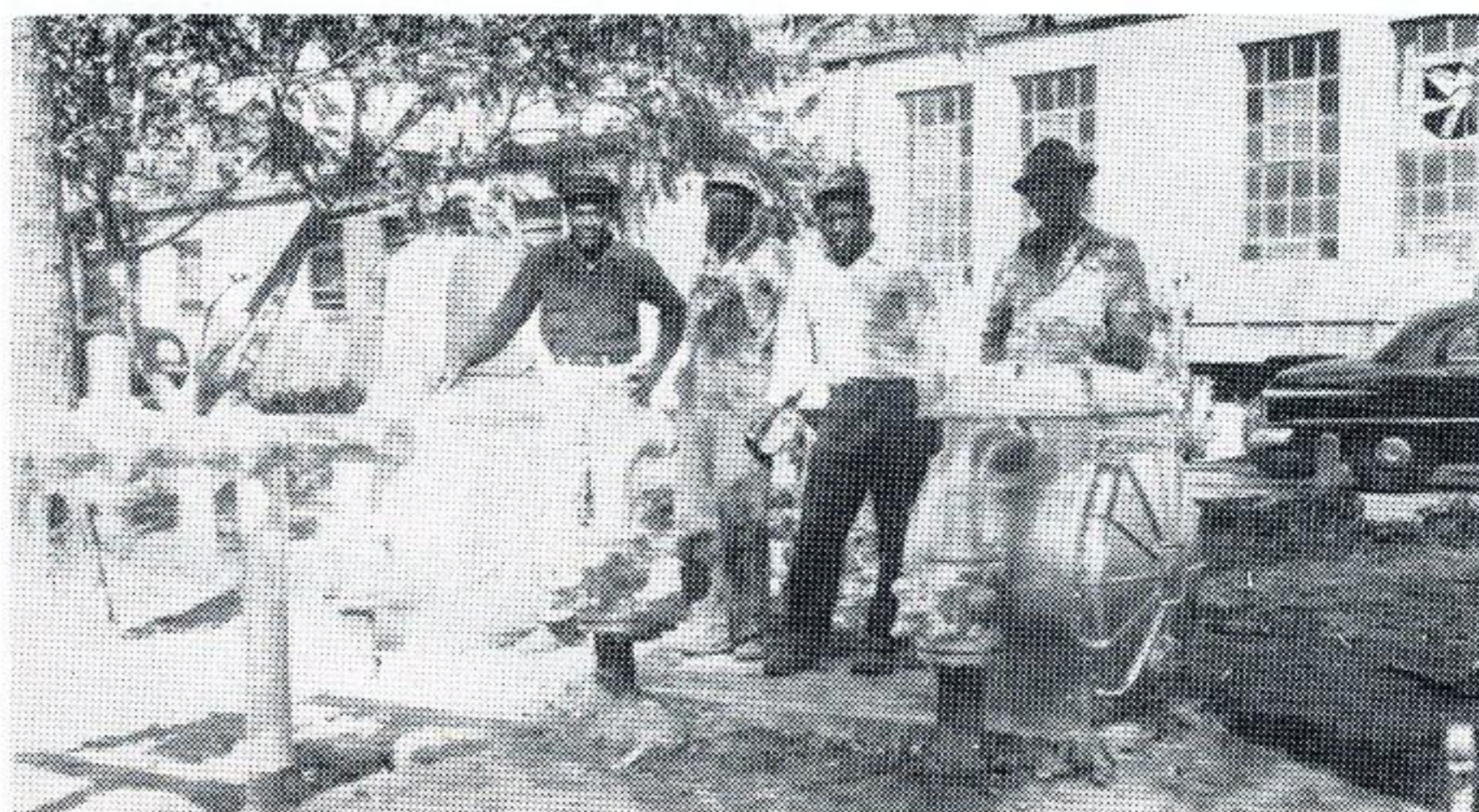
James Brooks, Louis Knighten, Jimmie Thornton and foreman Wallace of the gas department are shown after they set the hospital's new gas meter.
