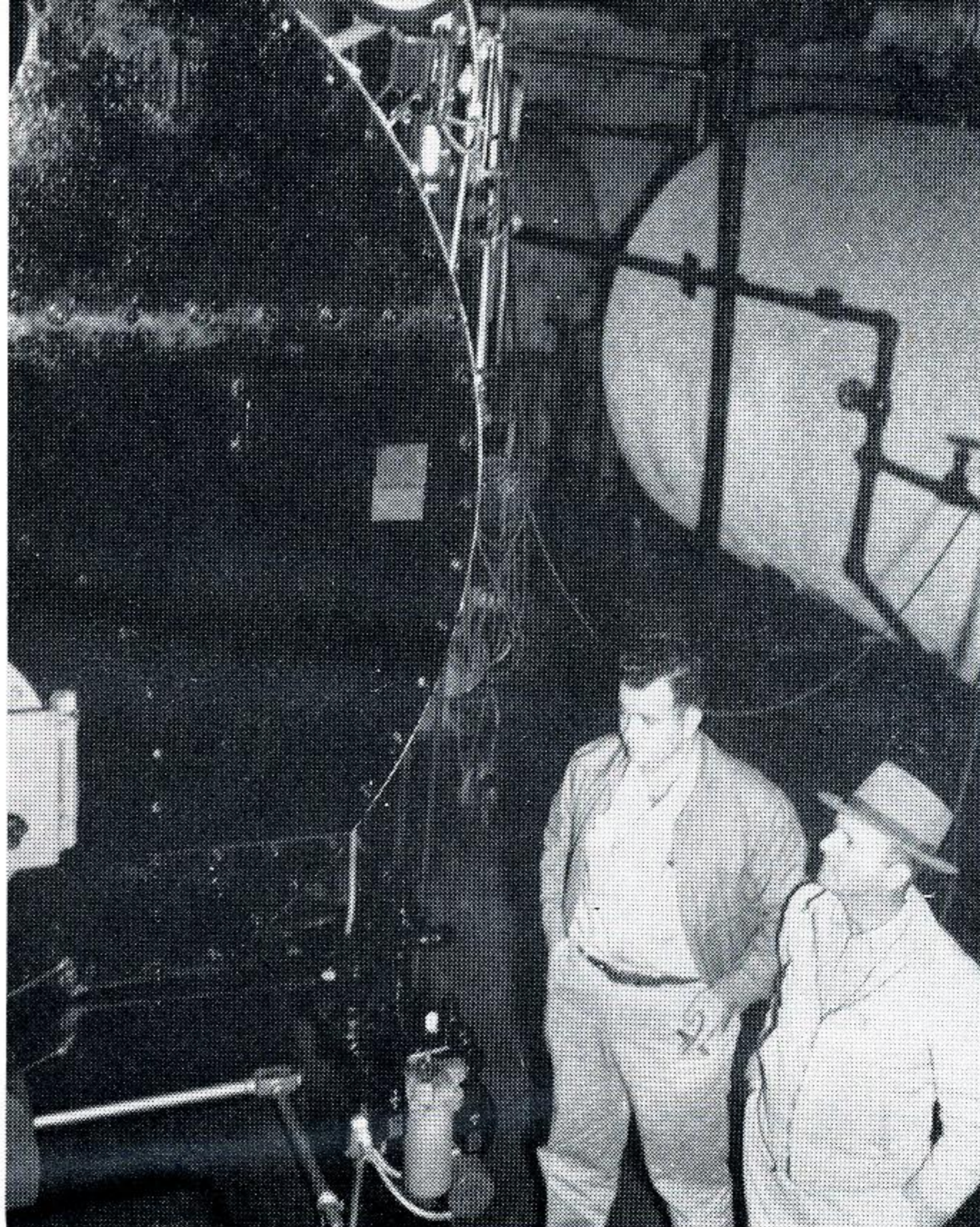
GSU labor foreman L. E. Wallace (right) is shown heavy-duty boilers, now fired with natural gas, by hospital staff-member Neal.
