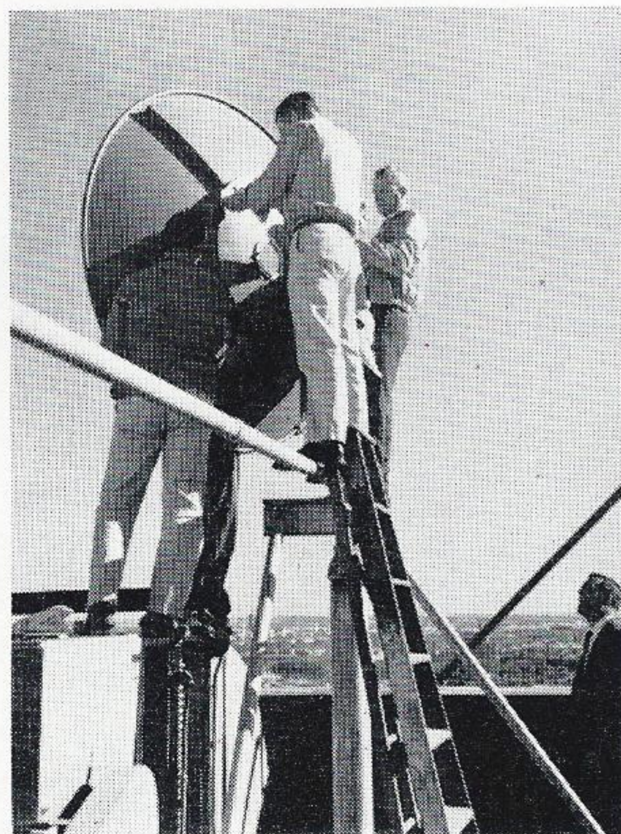
The microwave antenna is being installed atop our Beaumont Main Office Building by Willis Reed, W. Haack, communications technicians 3rd class, M. T. Alford, communications technician 2nd class, W. P. Tucker, relayman 1st class and J. M. Patterson, field engineer for the prime contractor for installing the system, Motorola Communications and Electronics, Inc. Haack is mostly hidden by the antenna.
