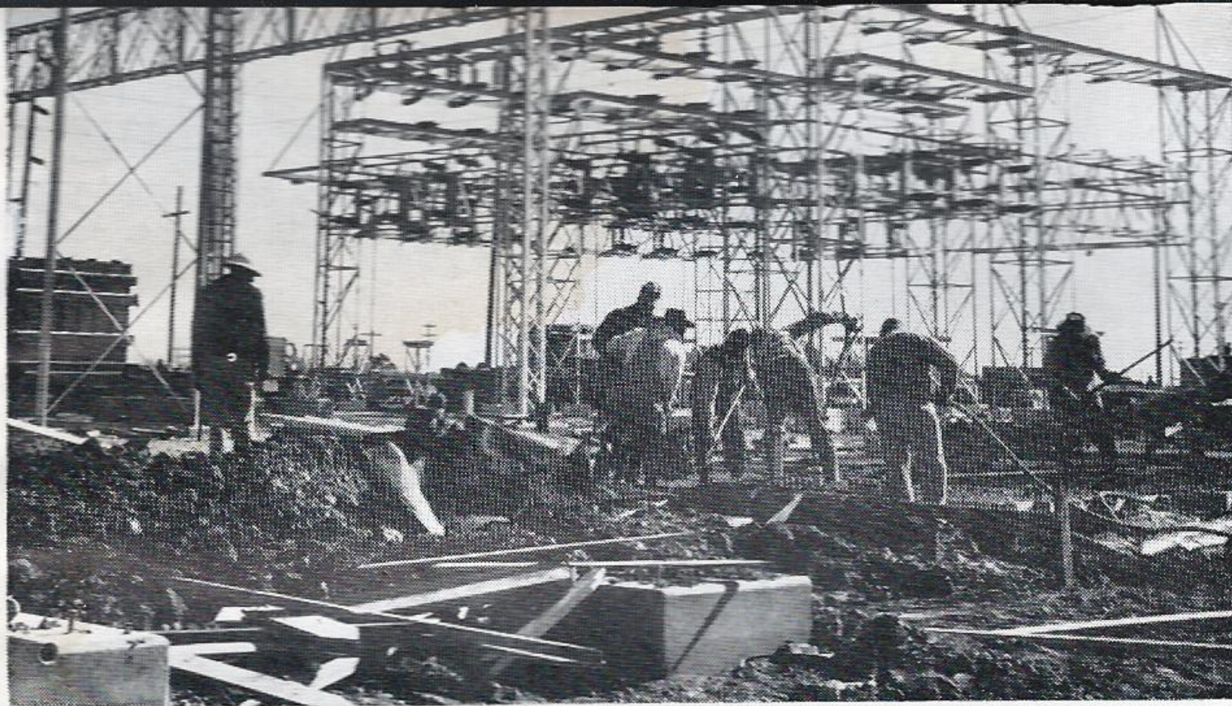
Many substations will be built or expanded this year.
