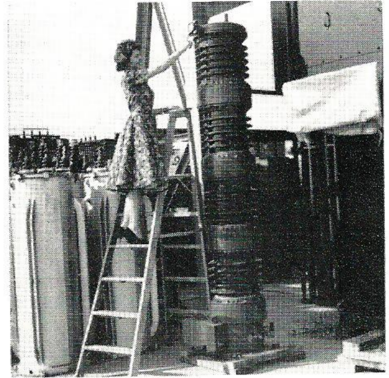
J. 138,000 primary voltage potential transformer
