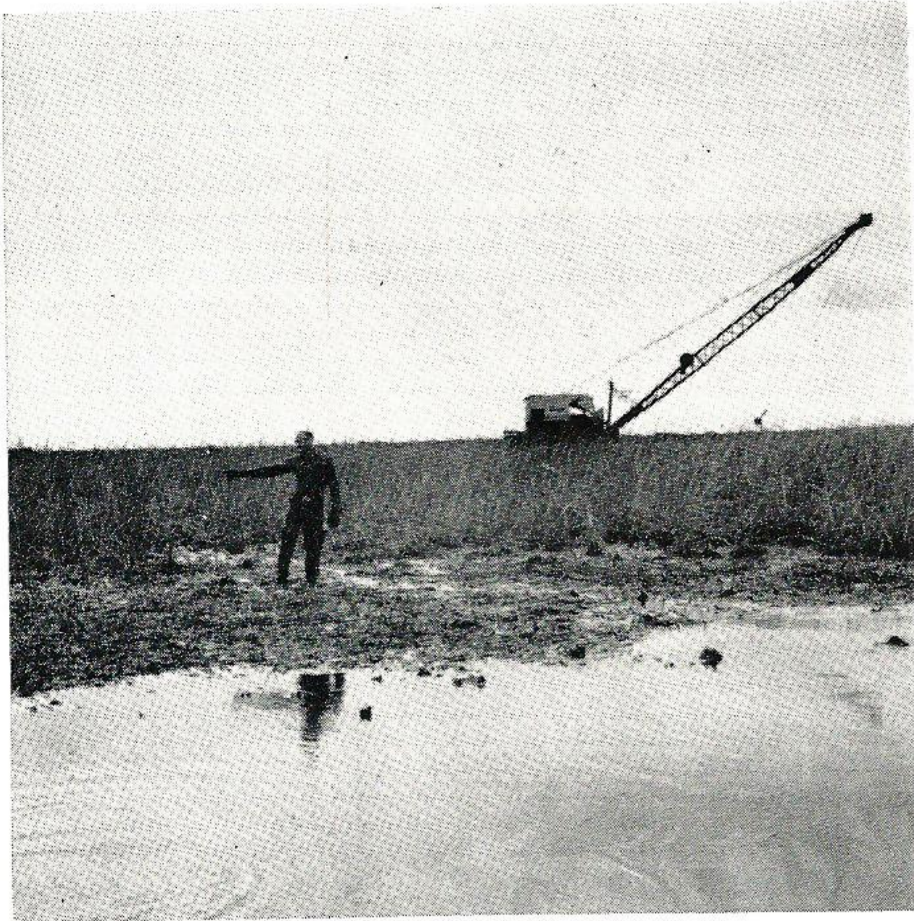
Dredging of the intake and discharge canals from Sabine Lake to the power station and from there to the Neches River is nearly complete. J. B. Hawkins, of the Moreland Dragline Company, points out the route he is following. So far, he's killed 17 water moccasins.
