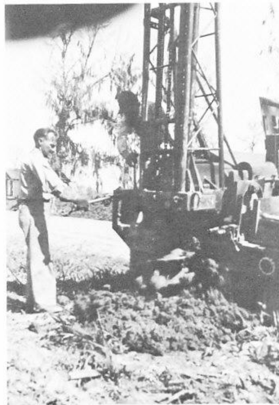
Phil LeVert, now a utility foreman in the Substation Department, Baton Rouge, digs a hole with the division's first mechanical hole digger. This was purchased in 1945.
