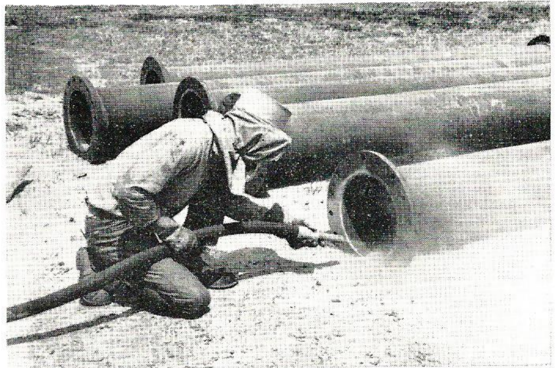
CLEANS PIPE. Ernest Meche of Trevor-Boyce, sandblasts a section of pipe in preparing it for rubber lining. Sandblasting under 80 lbs. pressure cleans the pipe's inner surface of rust, providing improved adherence of the rubber.
