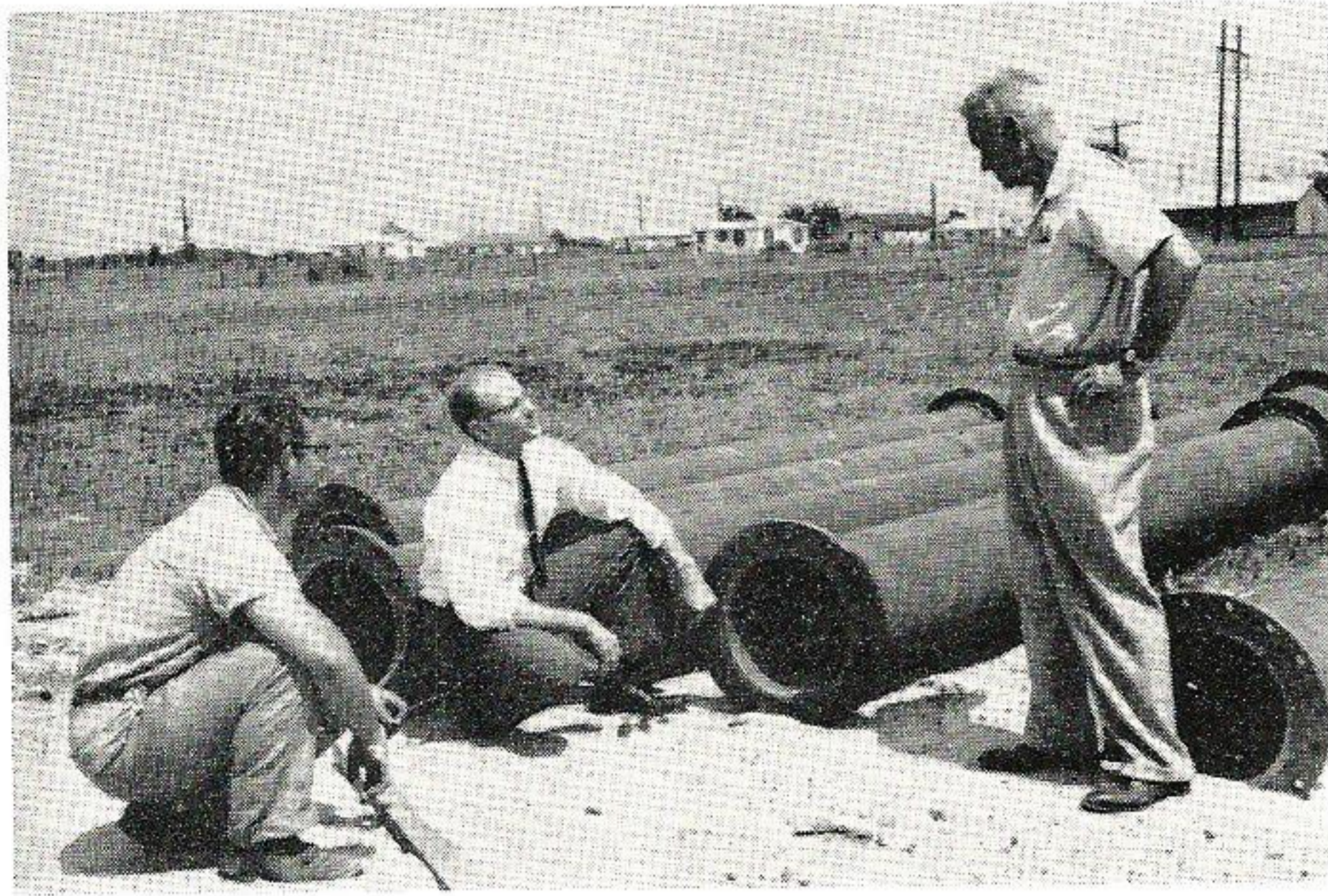
INSPECT PIPE. Ike Kolarik of Trevor-Boyce Associates; Aubrey Sprawls, area development engineer; and Curtis Lusk, local superintendent, Dayton, Texas, note the condition of pipe sections that are to receive a Triflex lining.
