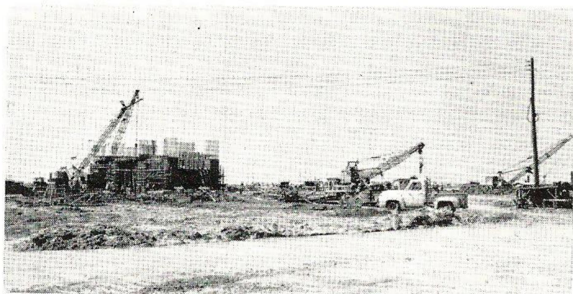
FOUNDATIONS TAKE SHAPE. Construction crews are on schedule at Sabine Station as the foundations for units one and two take shape.
