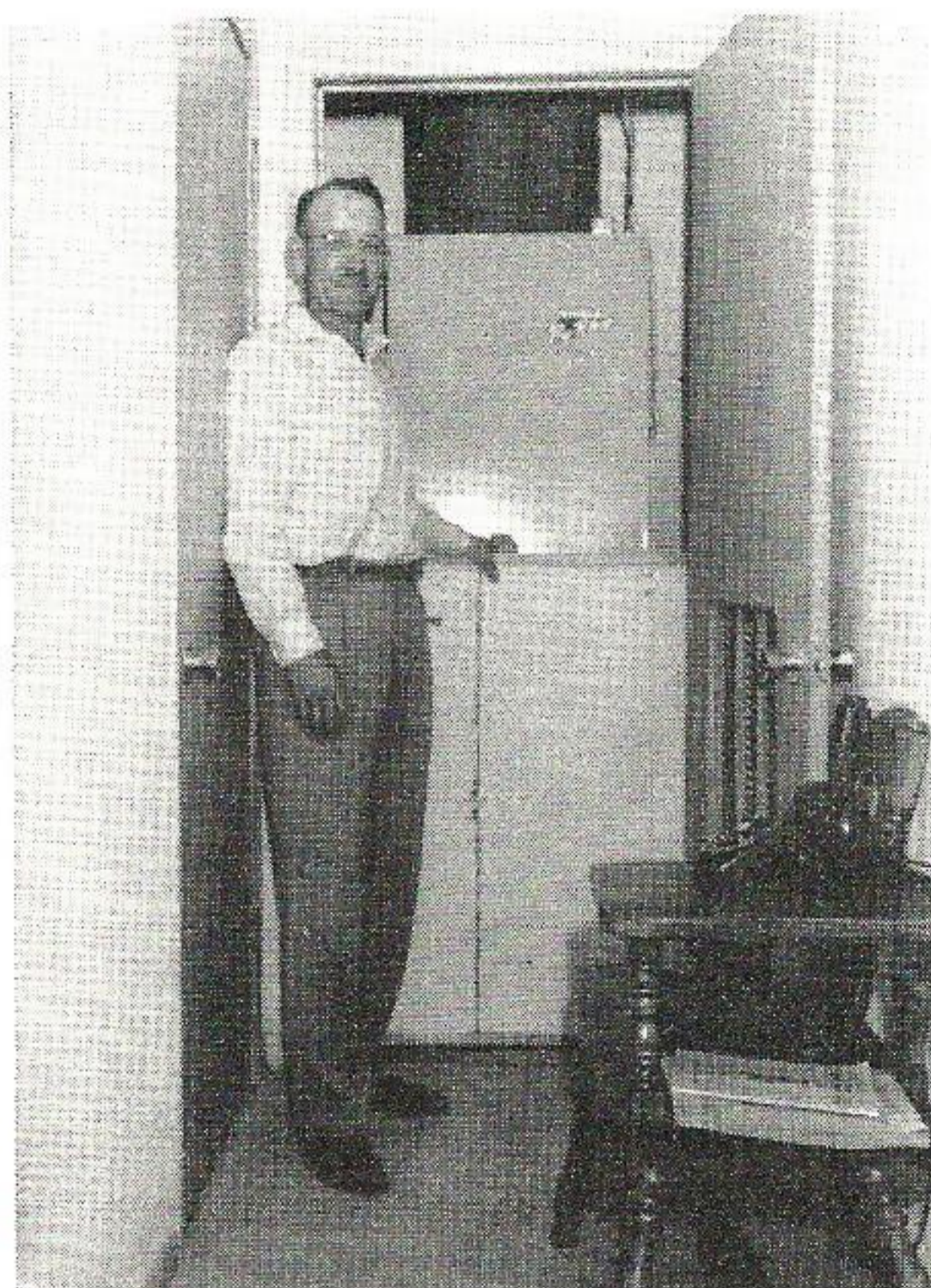
ENJOYS HEAT PUMP. Mr. Adams placed this acoustics board screen in front of his heat pump closet to lessen the noise, yet, it allows air to circulate around the pump.
