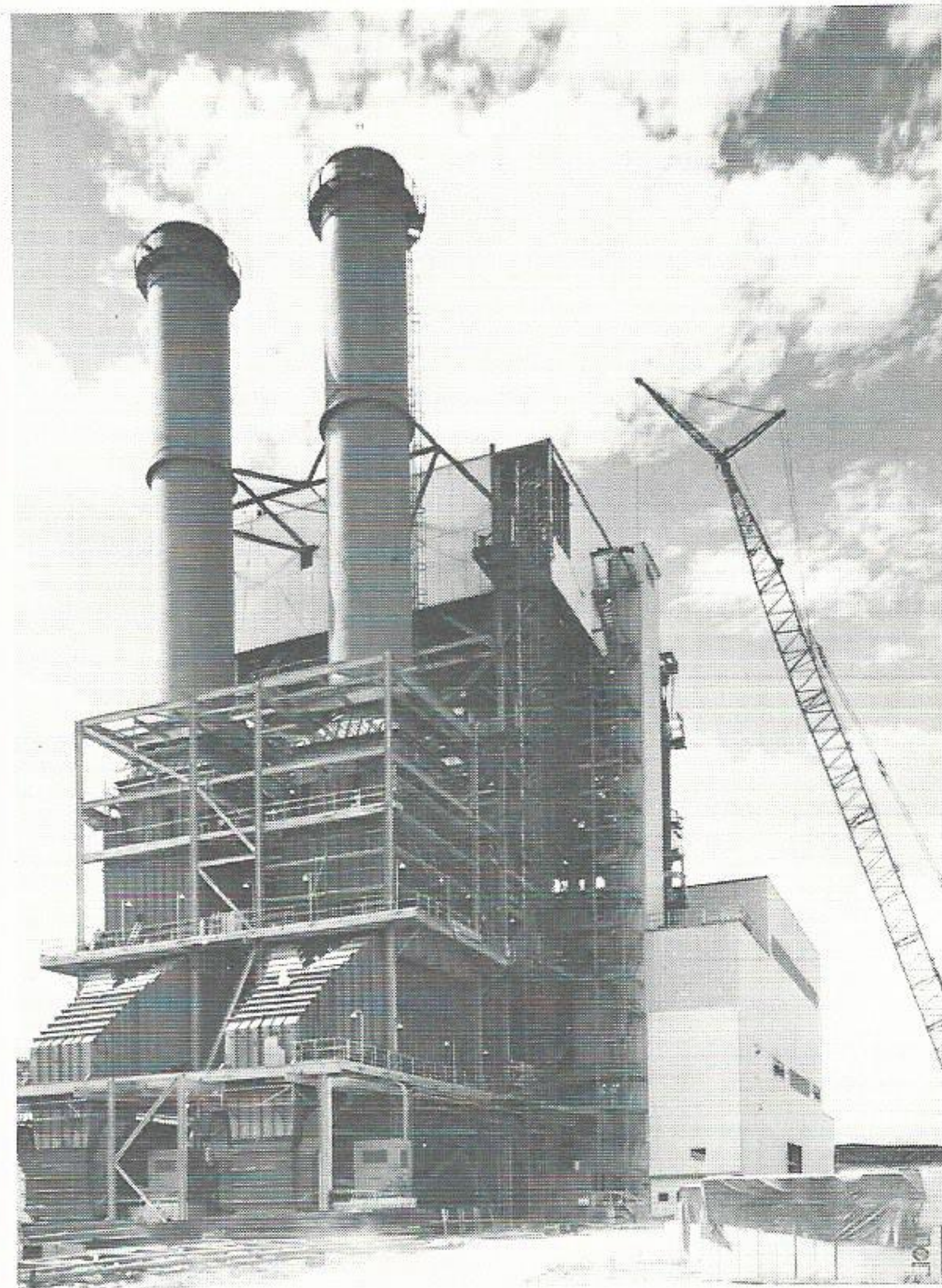
Ready to start generating kilowatts is the Number Four unit at Roy S. Nelson Station near Lake Charles. This 580,000 kilowatt machine boosts Nelson's capability to 964,000 kilowatts, making it our largest station until Willow Glen No. Four goes on the line.
