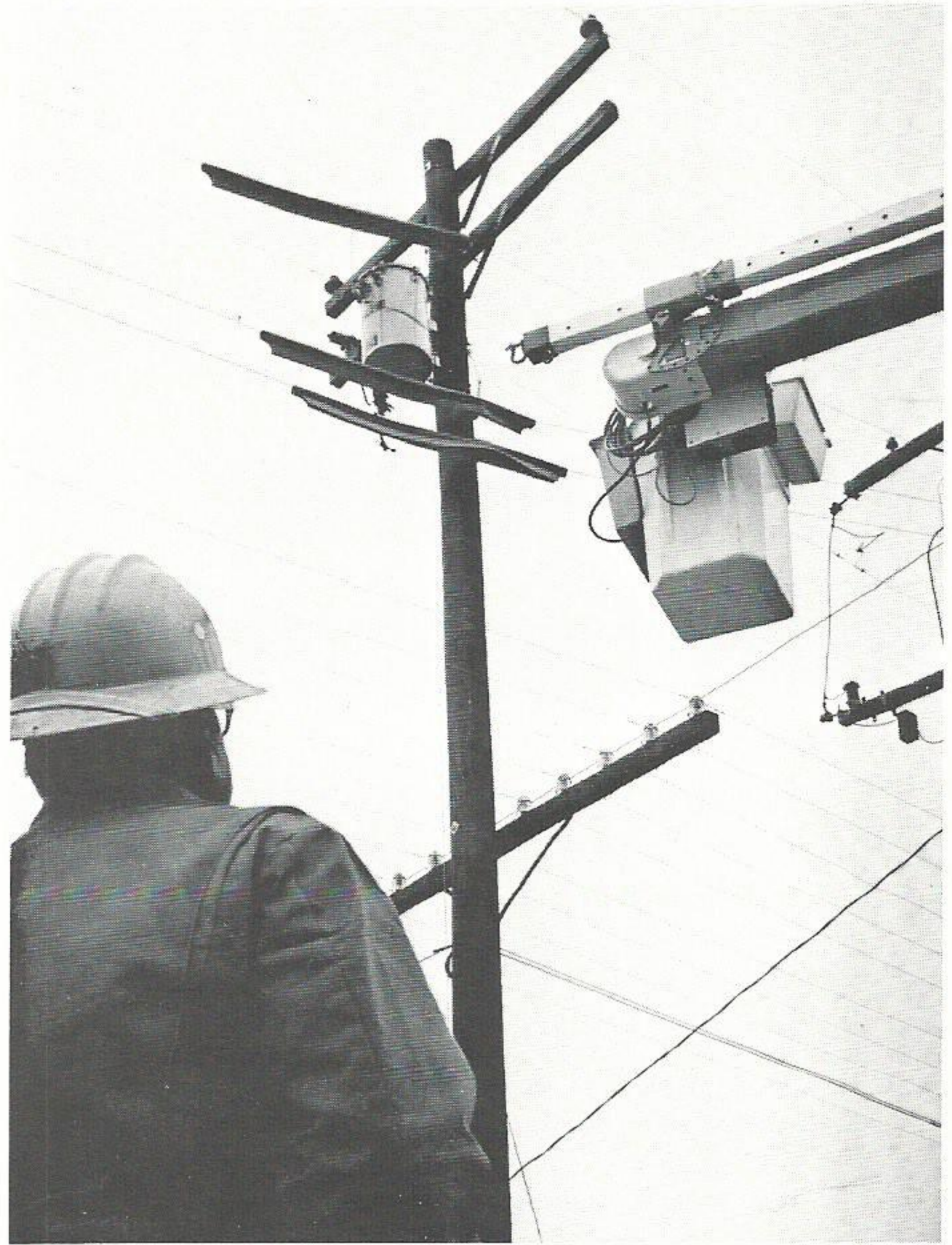
Below Lineman 1st Class Lem Gravelle (in bucket) prepares to change out wiring assisted by Helper Allen Broussard. Bruce watches the job preparations and above he helps guide Lem into position.
