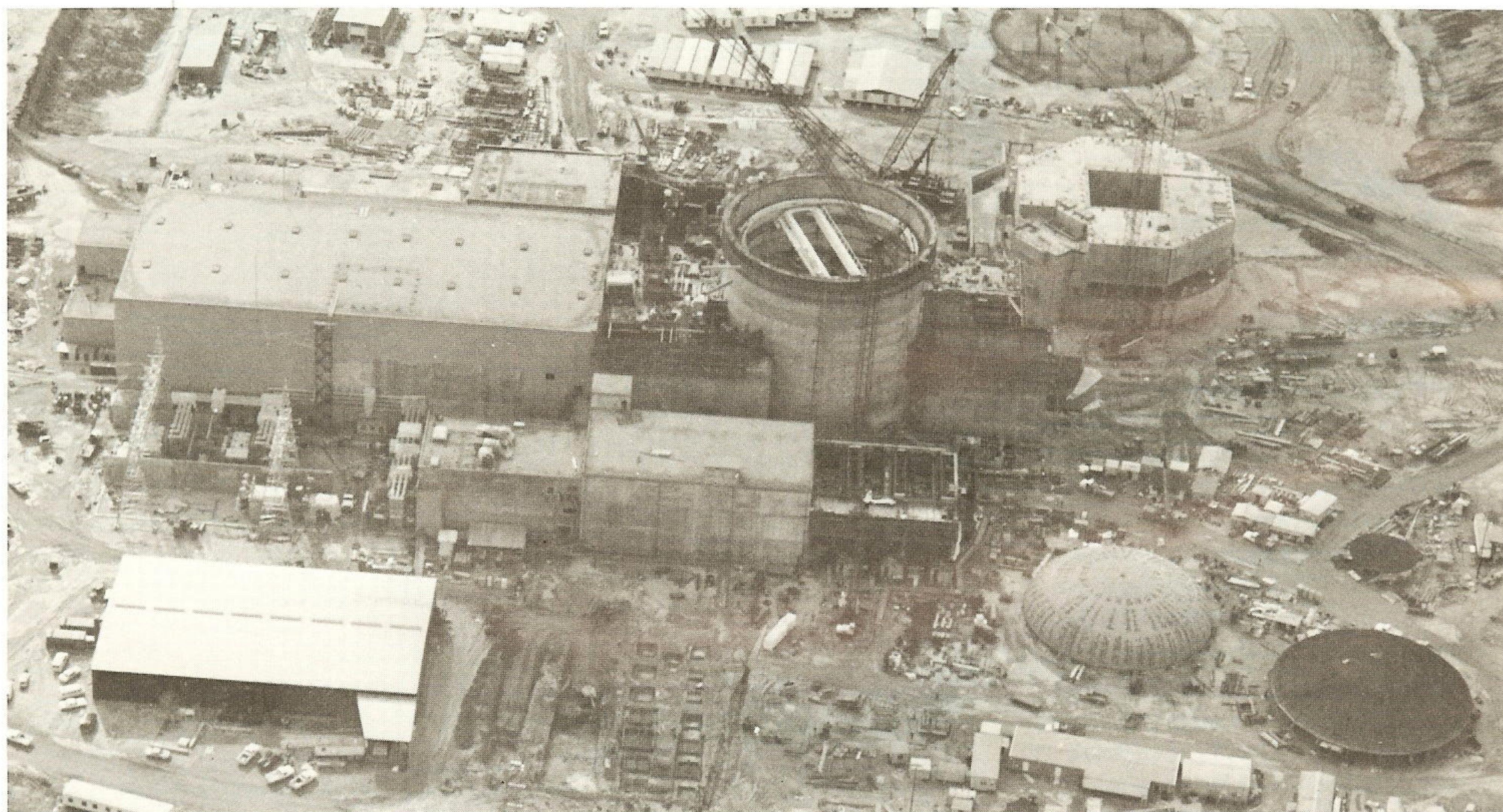
River Bend I will be GSU's first nuclear power plant.
