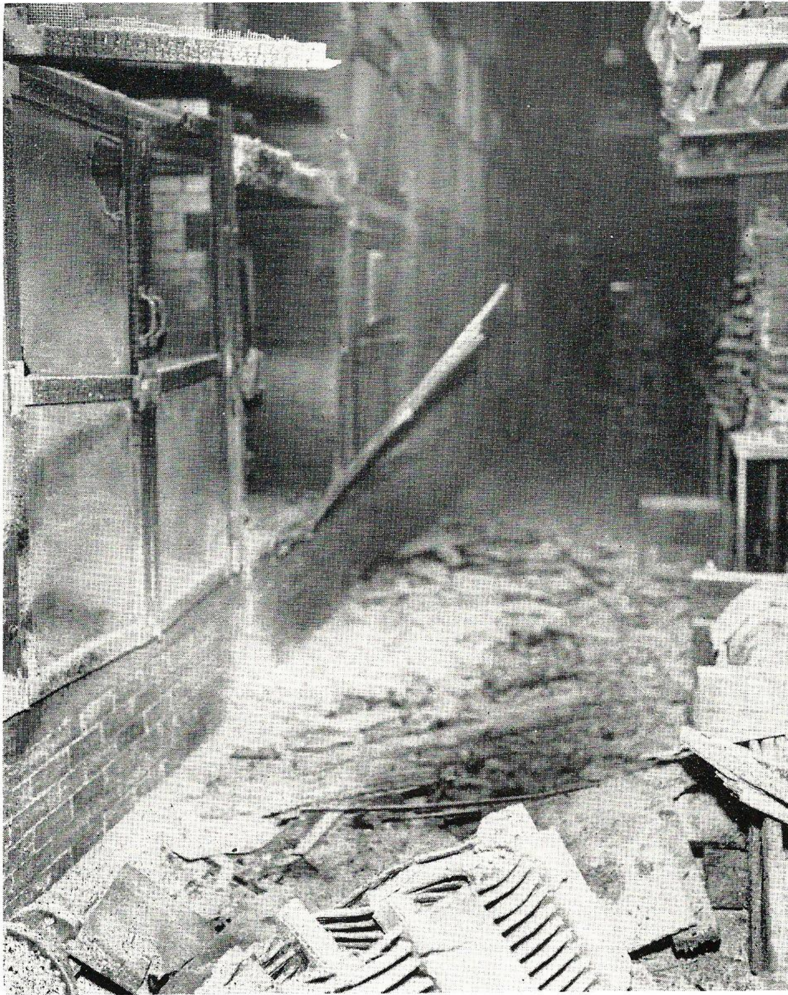
WHERE LIGHTNING STRUCK. Main 13 kv feeder and reactor buss room looked like this after lightning bolt struck. Picture was taken at midnight by Jack Worthy.
