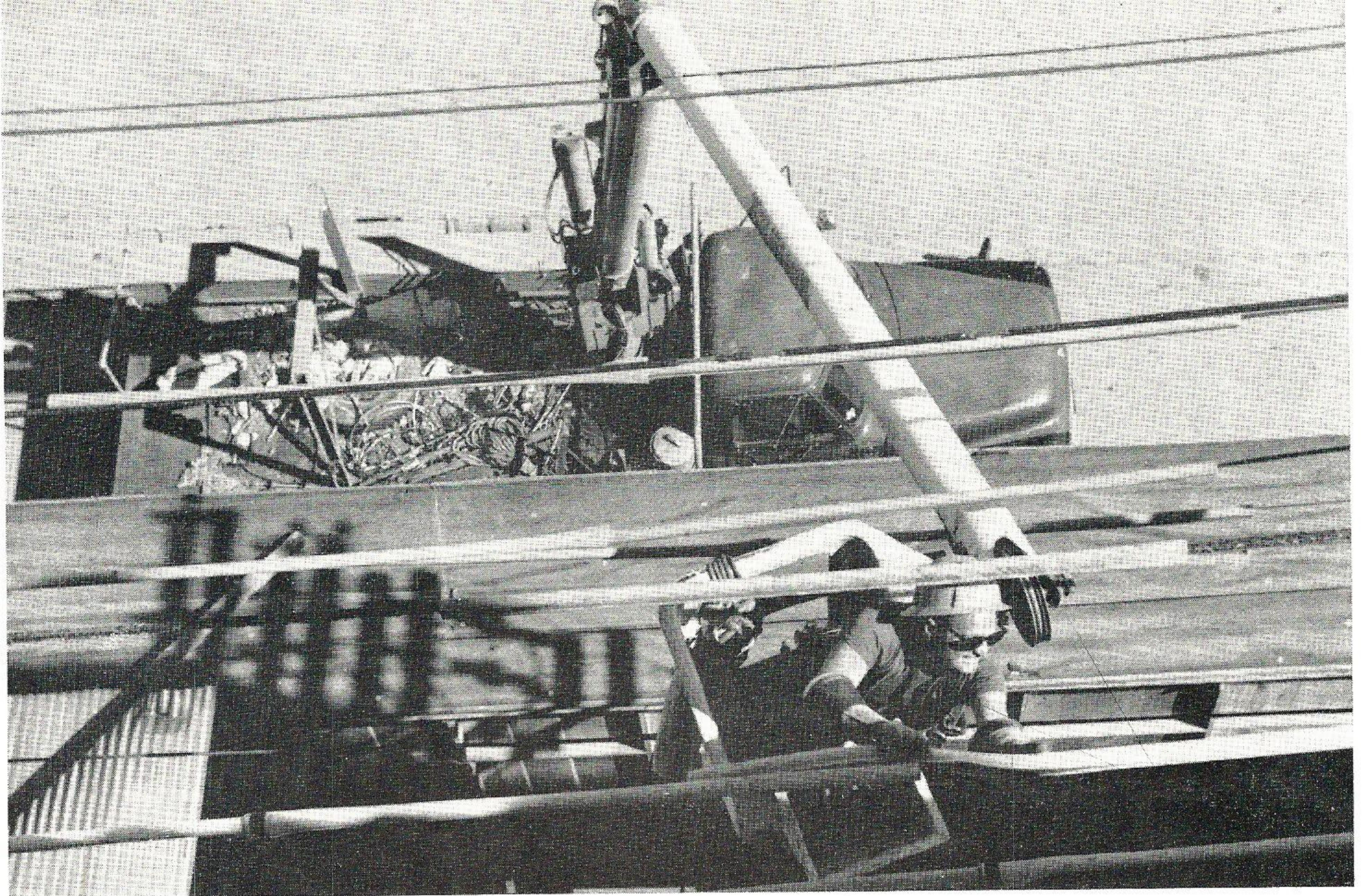
P. E. Sanderson, Line Department, Beaumont, utilizes the extended reach of the "Apple Picker" to cover wires alongside the Beaumont Enterprise and Journal building. The building is being remodeled and the rubber "gut" covering will protect workers.
