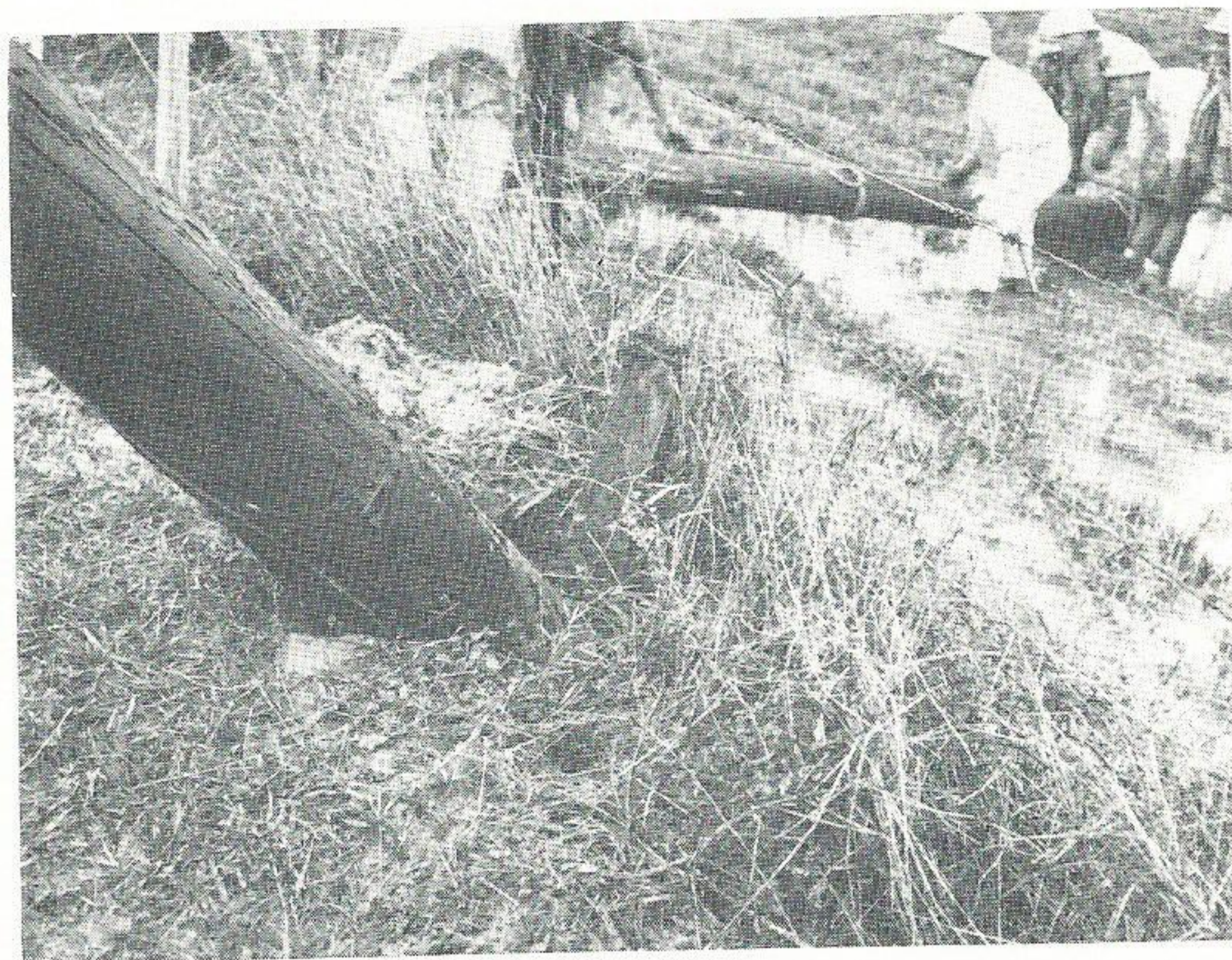
REPAIR DAMAGE. Service crews of the Lake Charles Division work long and hard to rapidly restore service to areas struck by the tornadic winds and heavy rains on March 17. Here a line crew is replacing a pole which was downed by the wind west of Lacassine.
