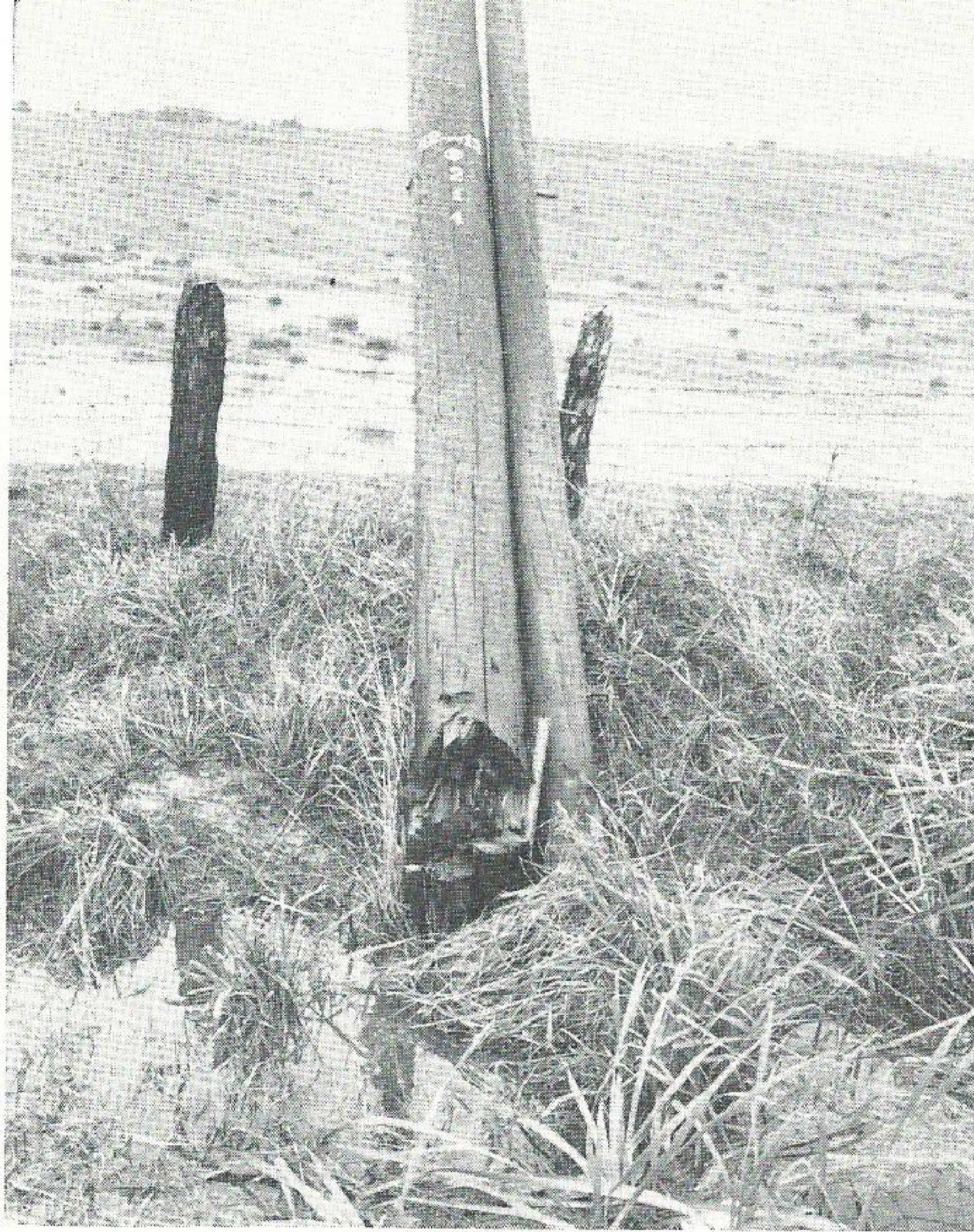
POLE DAMAGE. This structure was broken by a small tornado which skipped along U.S. Highway 90 west of Lacassine. A number of structures were downed in this area.
