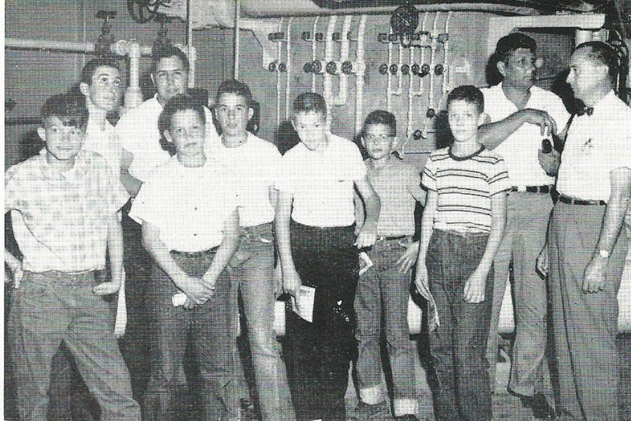
4-H GROUP VISITS WILLOW GLEN. Eight students enrolled in the electric project of the Riverside 4-H Club of Baton Rouge toured the facilities at Willow Glen Generating Station
