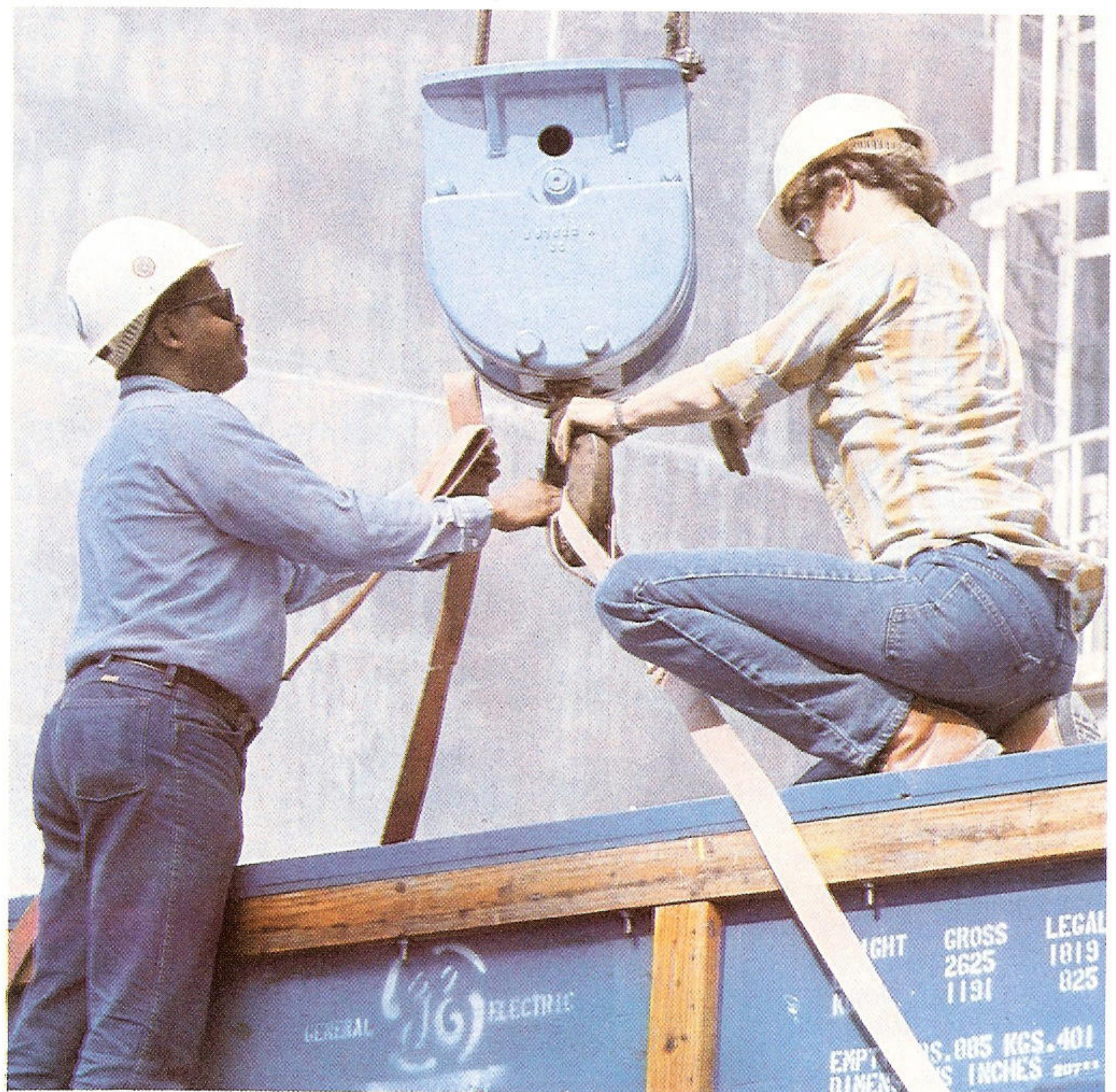
Joe Jones and Joe Martin, repairmen-1st class-nuclear, attach a hook to a box of fuel bundles prior to unloading.
