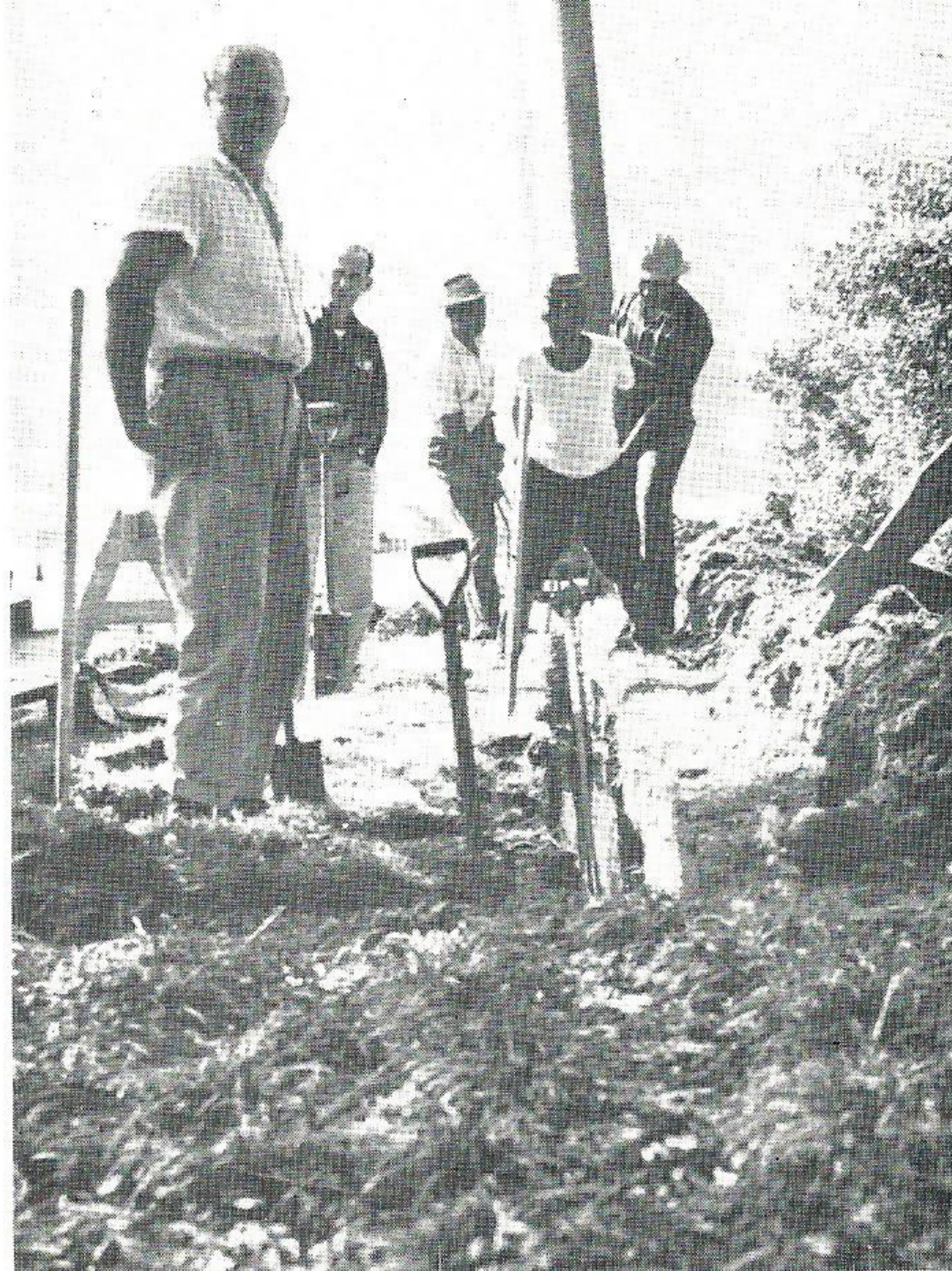
REPLACING OLD PIPE. A 31-year old gas main in an older part of the city is replaced with newer pipe by Foreman F. Van Busch (in foreground), and his crew. Behind Mr. Busch is M. L. Day, engineering assistant. Crew is using a power-driven water boring machine to bore a hole underground to avoid tearing up planted surface—which helps maintain good public relations for our Company.
