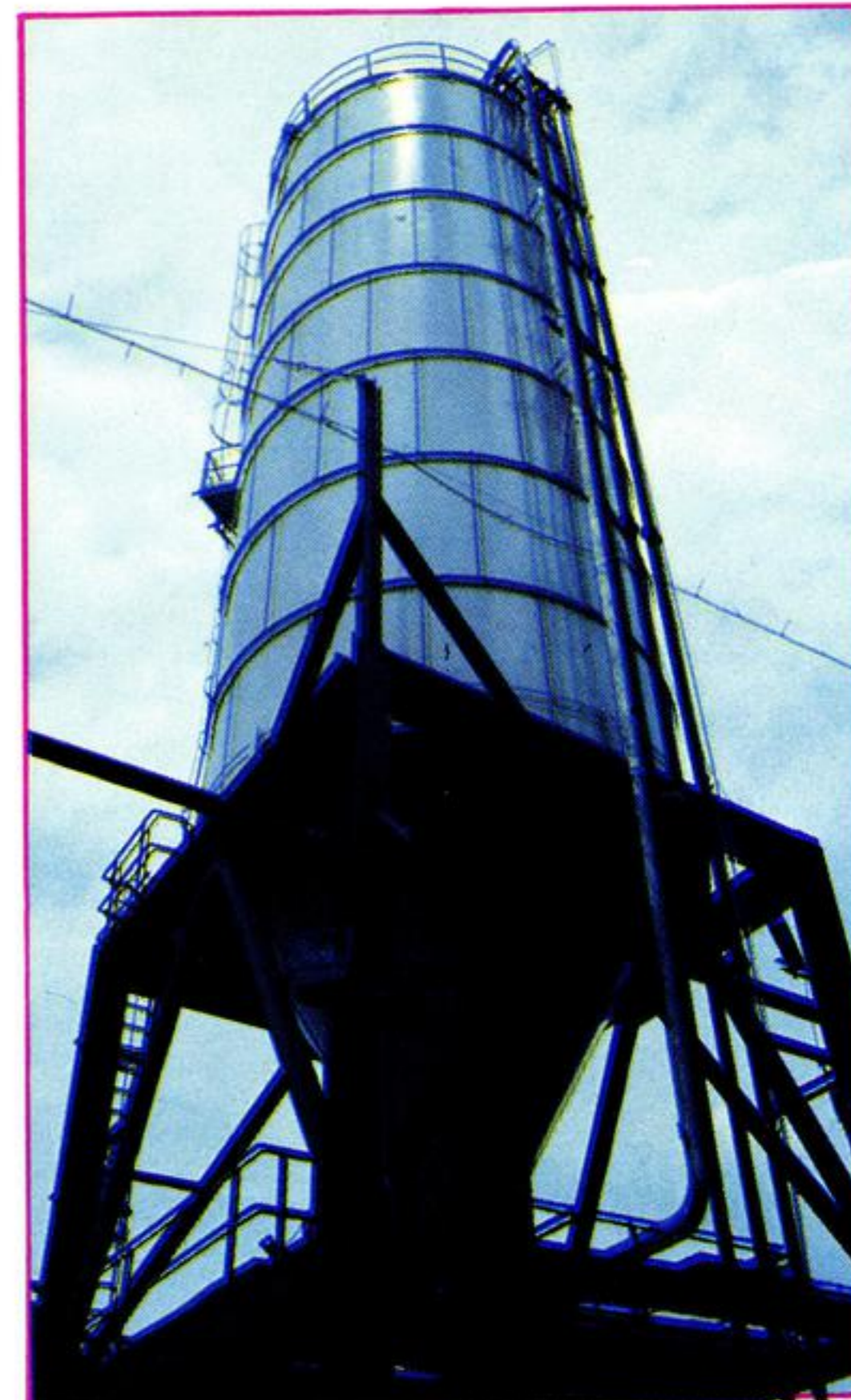
Rice ash, stored in this hopper, will be used as insulation material.
