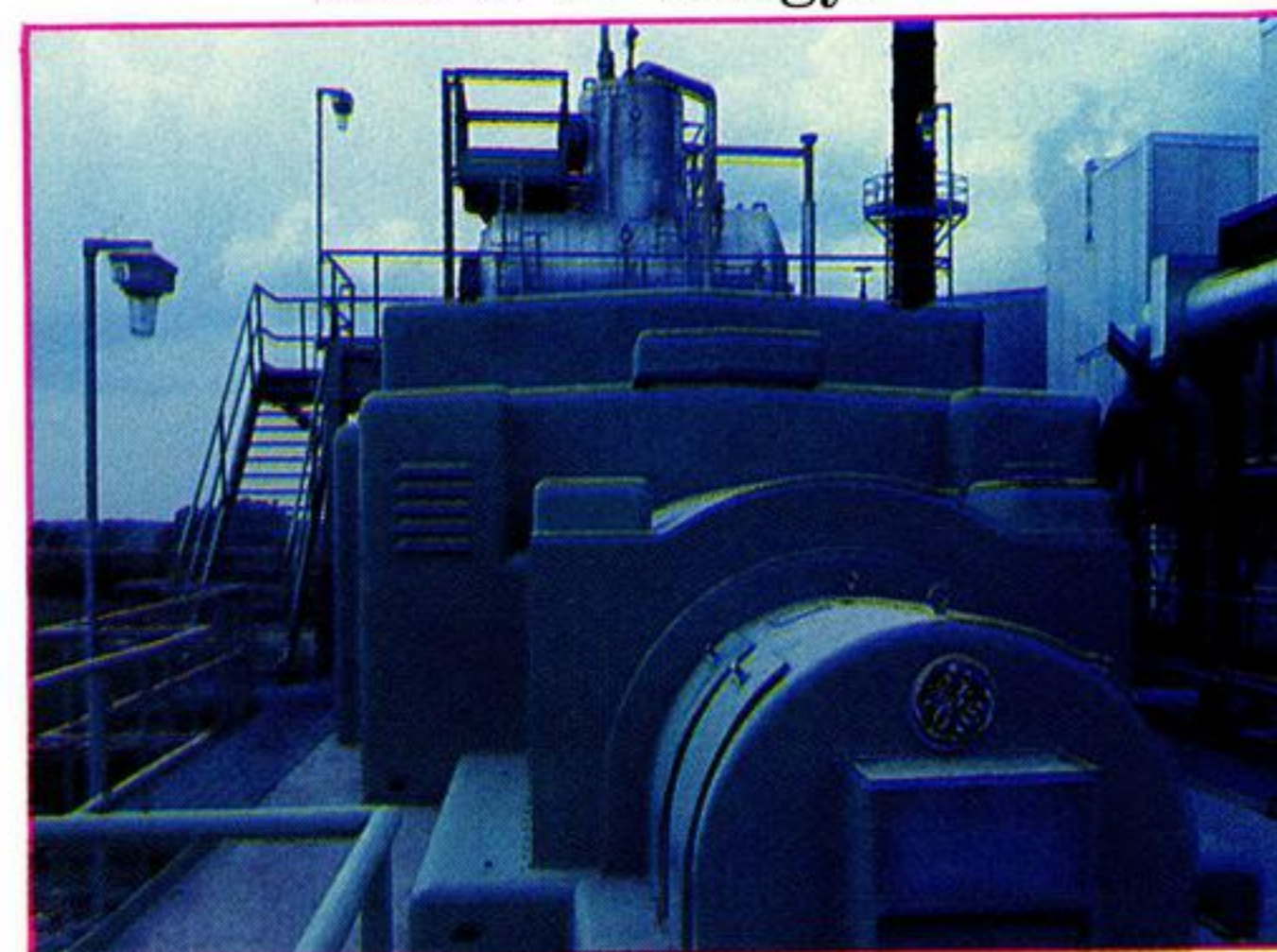
A large generator produces the power that is sold back to GSU.
