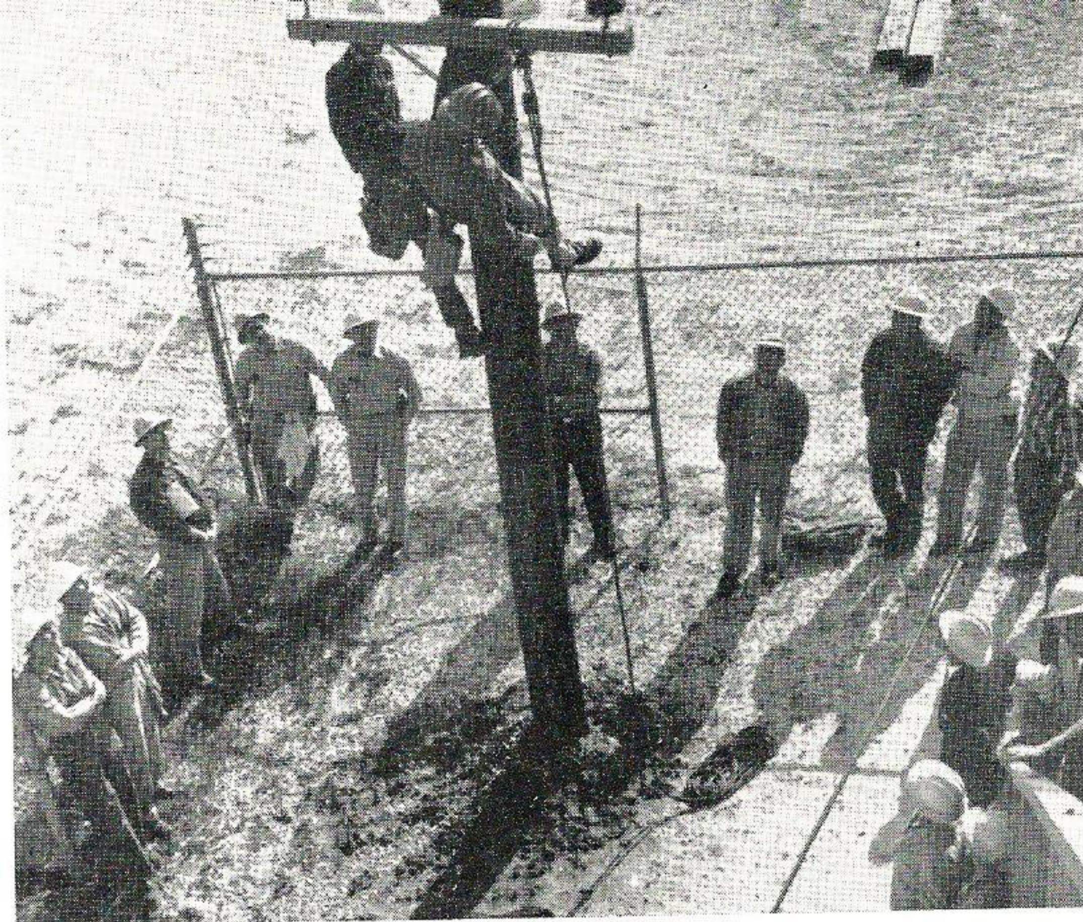
EXCHANGE KNOWLEDGE. Members of the Baton Rouge Line and Safety Departments instruct the plant electricians of the Baton Rouge Works of Kaiser Aluminum and Chemical Corporation in the techniques of rescuing an injured man from the top of a hot pole. Picture from THE ALUMINATOR, company newspaper for the Baton Rouge Works.
