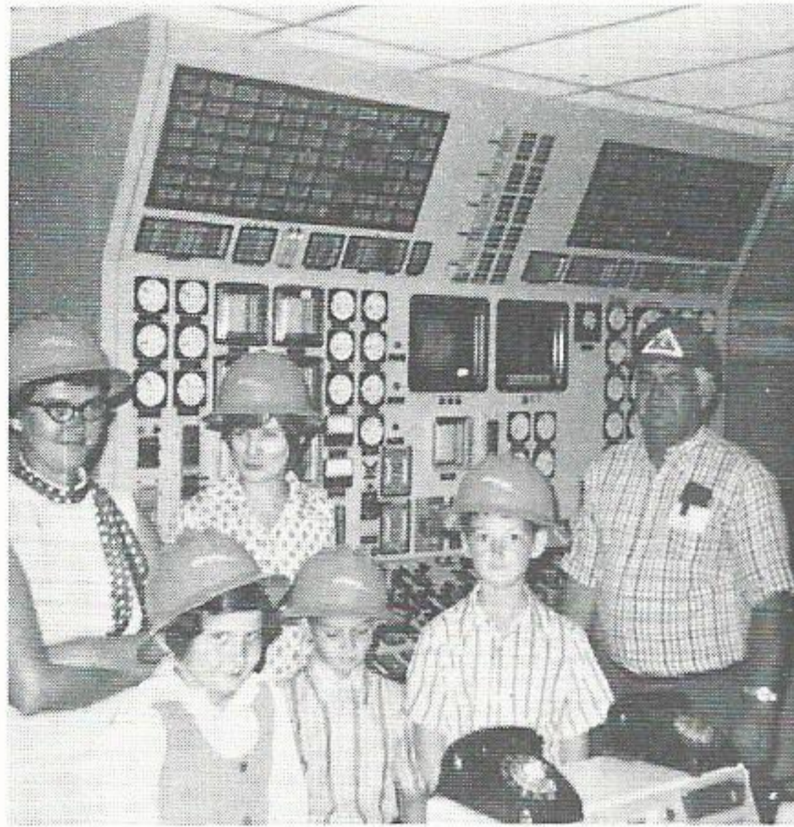
The Port Arthur Sales Department recently had a tour of Sabine Station along with their families. Power plant personnel divided up the group and each took a certain number through the sprawlin facility. L. E. Stough, test maintenance foreman, is shown here with one group. From left to right in the control room are, Mrs. Tom Clark, Mrs. Sue Williams and their children, Pamela Sue Williams, Cary Clark and Craig Clark.
