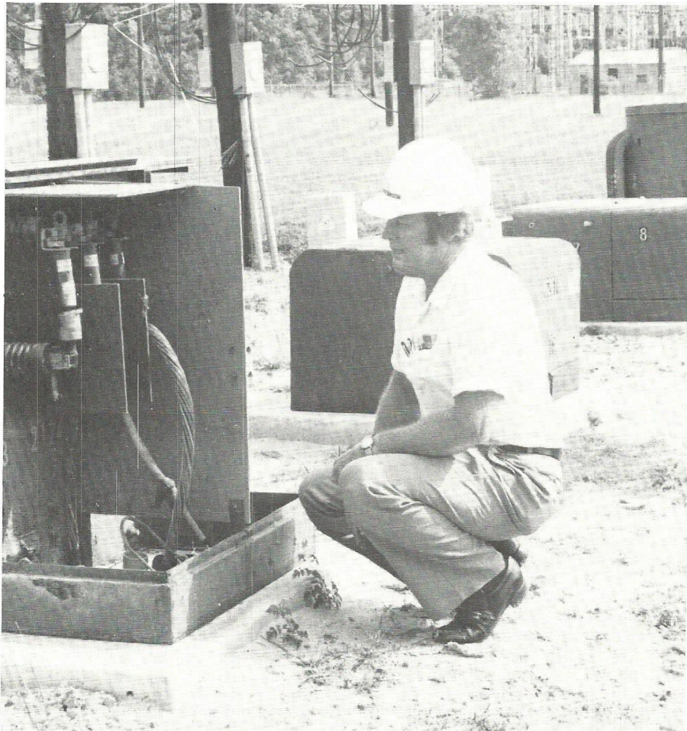
Butch Coon examines the workings of a pad mount transformer.
