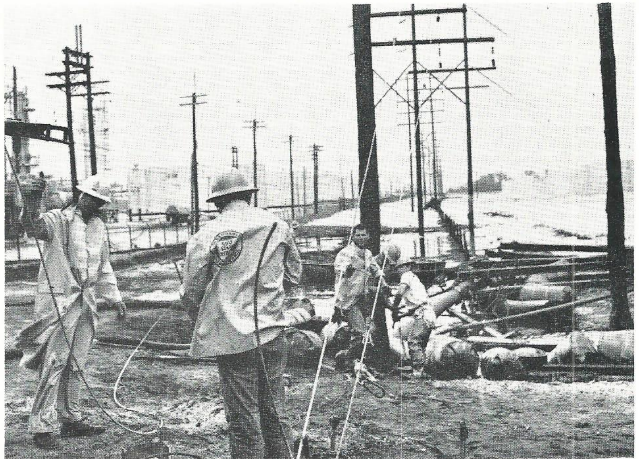
LAKE CHARLES HELPS BEAUMONT. Members of M. D. Byrd's line crew from Lake Charles are shown repairing our lines across Beaumont's Mobil Refinery tank farm. The line, which served parts of downtown Beaumont, was burned down about midnight September 11 when gas and oil floating atop the flood waters ignited. Crew members are J. A. Troille, A. Landry, E. F. Heard, G. R. Hayes, R. R. Gibson, Everett Chamberlain, J. C. Benoit, and L. N. Saltsman.
