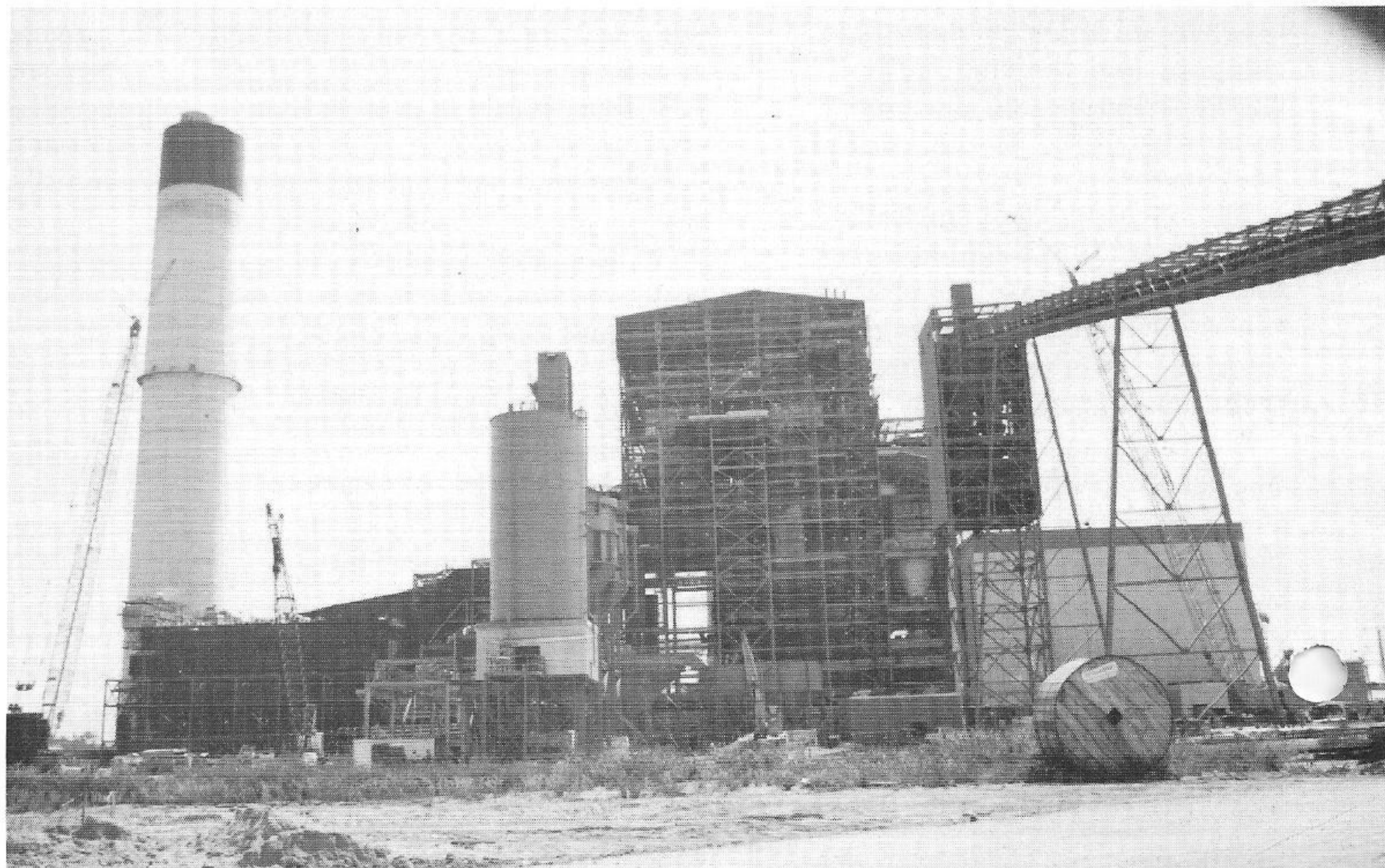
This view of Nelson 6 construction shows the 500-foot-tall chimney (at left) designed to house two independent brick flues — one for Nelson 6 and another for Nelson 5, a second 540 megawatt coal unit tentatively scheduled to go into operation by April, 1987.
