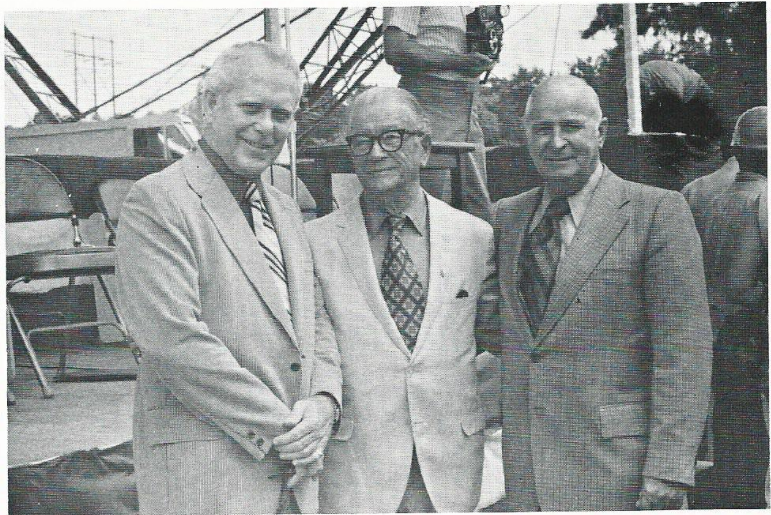
Just two weeks before his death, United States Senator Allen J. Ellender (D-La.) posed for the PLAIN TALKS camera during ground breaking ceremonies for a new bridge over the Mermentau River near Lake Arthur, La. The senior senator was seeking his seventh term in office. He was the only Louisiana congressman ever named President Pro-Tem of the Senate, and chaired the Senate Appropriations Committee. Flanking Senator Ellender are Joe Bondurant, left, manager of the Lake Charles Division, and Hutt Reed, Superintendent of the Jennings District.
