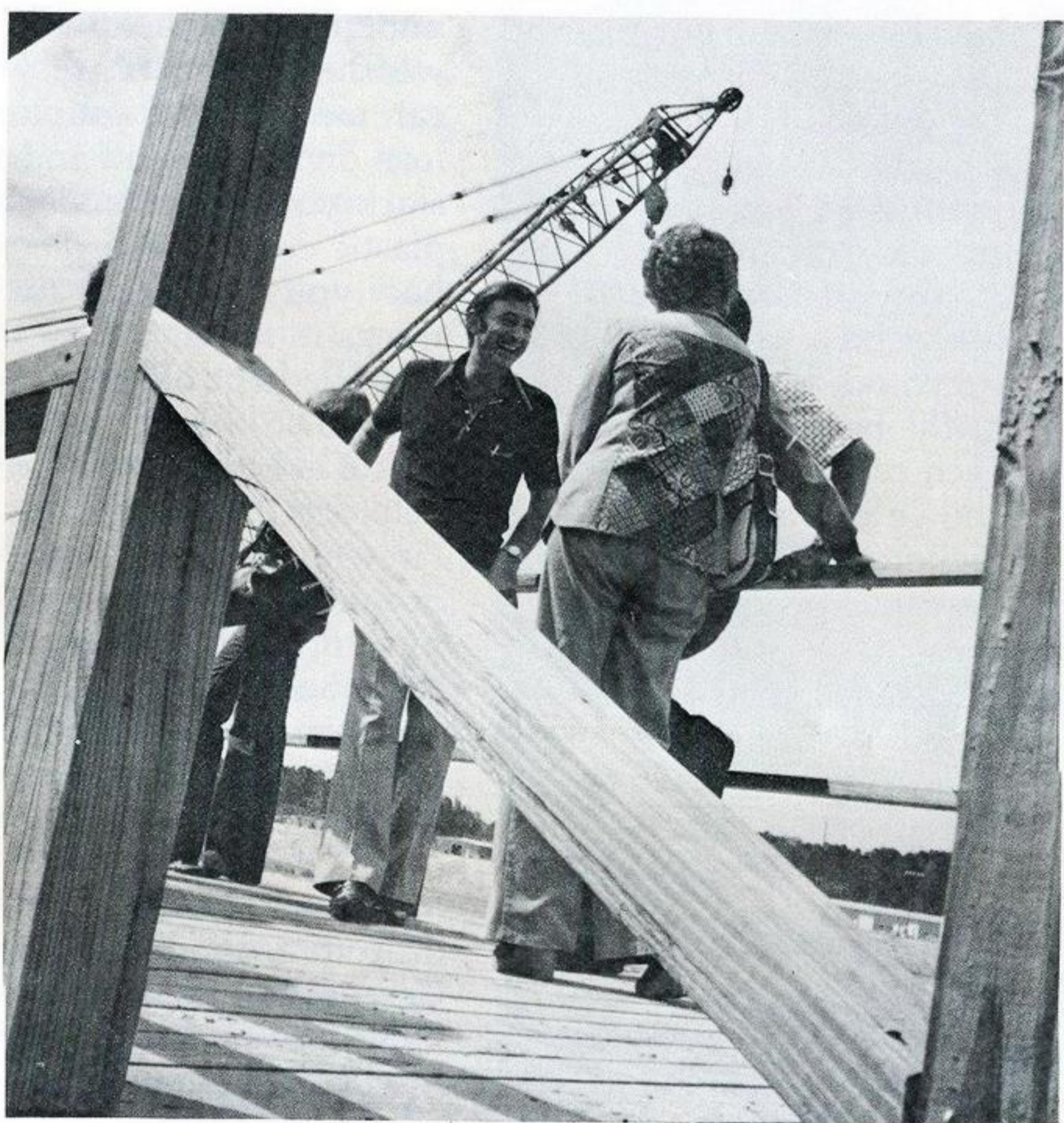
Some 75 persons took advantage of the company-sponsored tour on August 25 and got a mini-education in the workings and construction of a plant.
